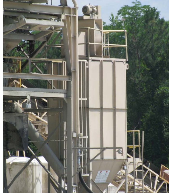
Central Dust Collector
