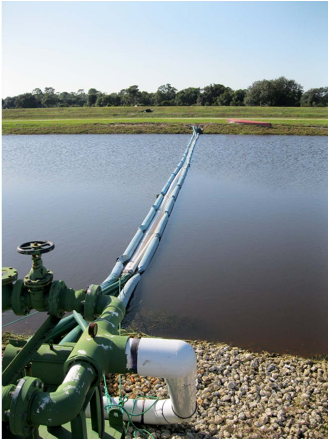
Figure 79. The eastern Grassy HWTT settling pond, with floating “floc line” that conveys wet floc from the contact ponds to the drying bed.
