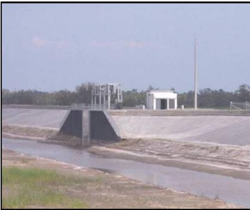
Figure 2-4. Intake structure and related facilities for S-383.
