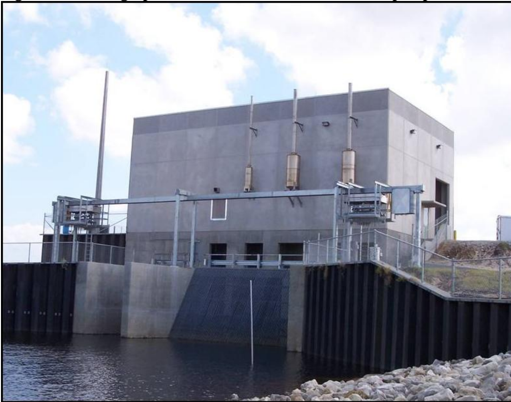
Figure 2-1. Photograph of the headwater side of the S-382 pump station.
