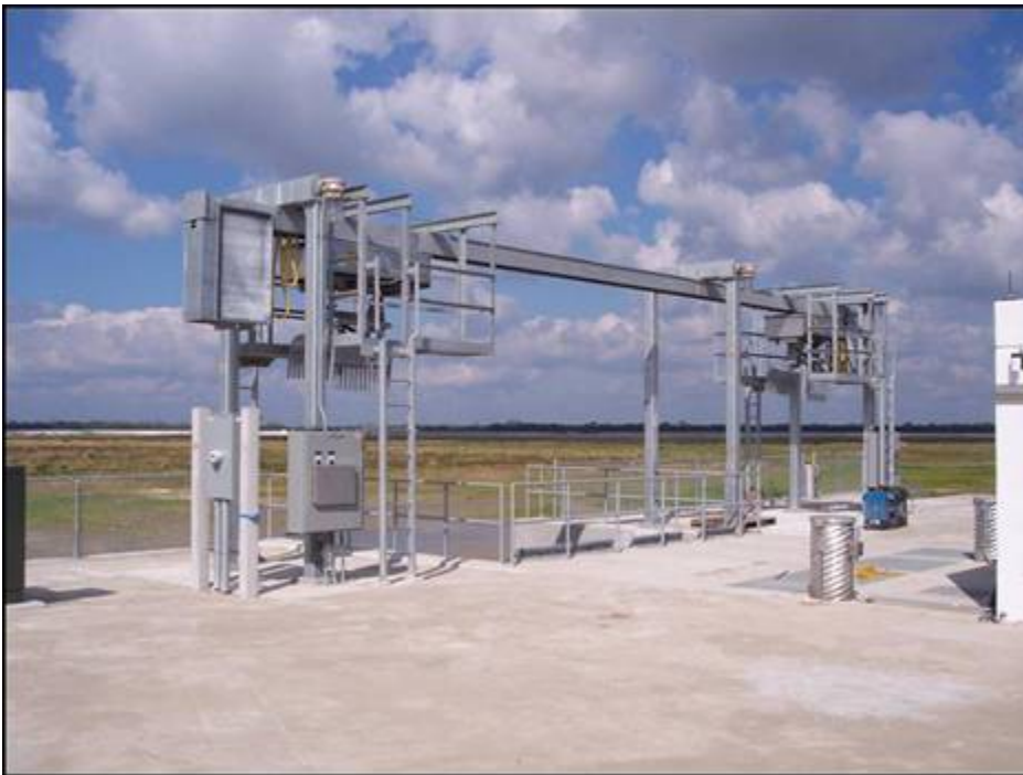
Figure 2-9. Trash rake monorail system for the intake bays at S-383.
