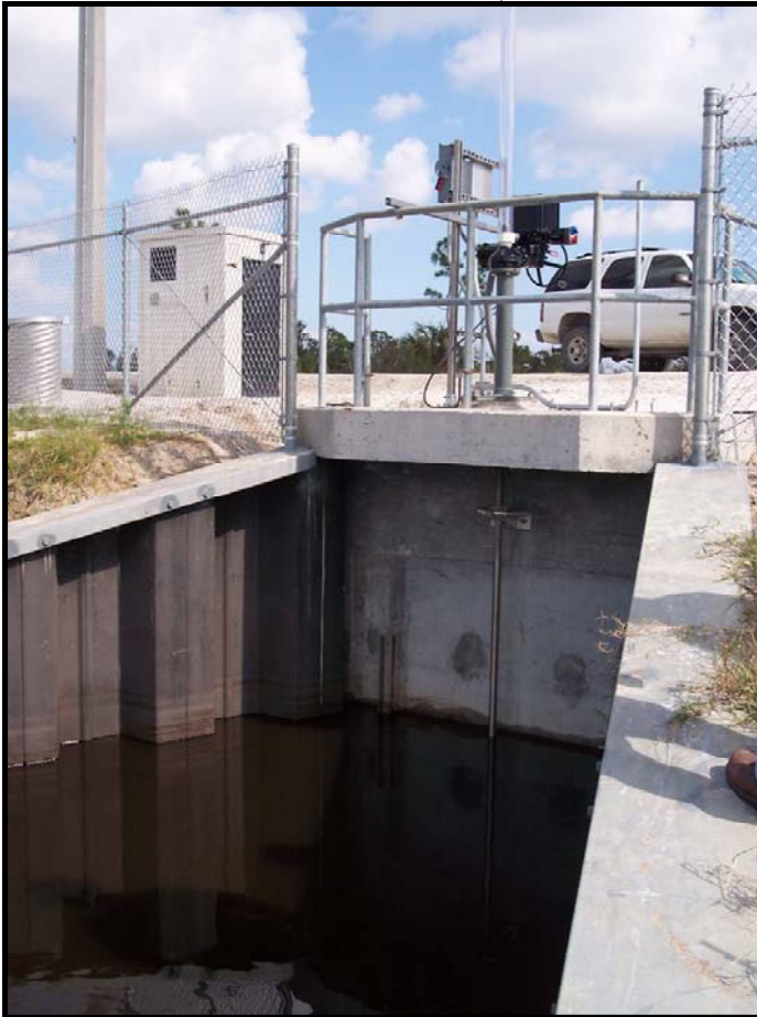
Figure 2-10. Photograph of the headworks of S-384 and Rating Curve for S-384 Under Low Head Difference Condition (from PBSJ 2002c).
