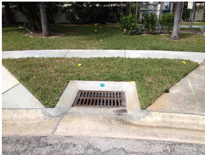
FIGURE 16: CITY OF INDIAN HARBOUR BEACH INLET AT HAWTHORNE COURT WEST AS PART OF THE LIME BAY EXFILTRATION PROJECT
