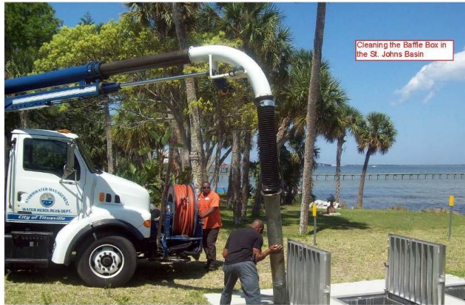
FIGURE 13: CITY OF TITUSVILLE BAFFLE BOX CLEAN OUT
