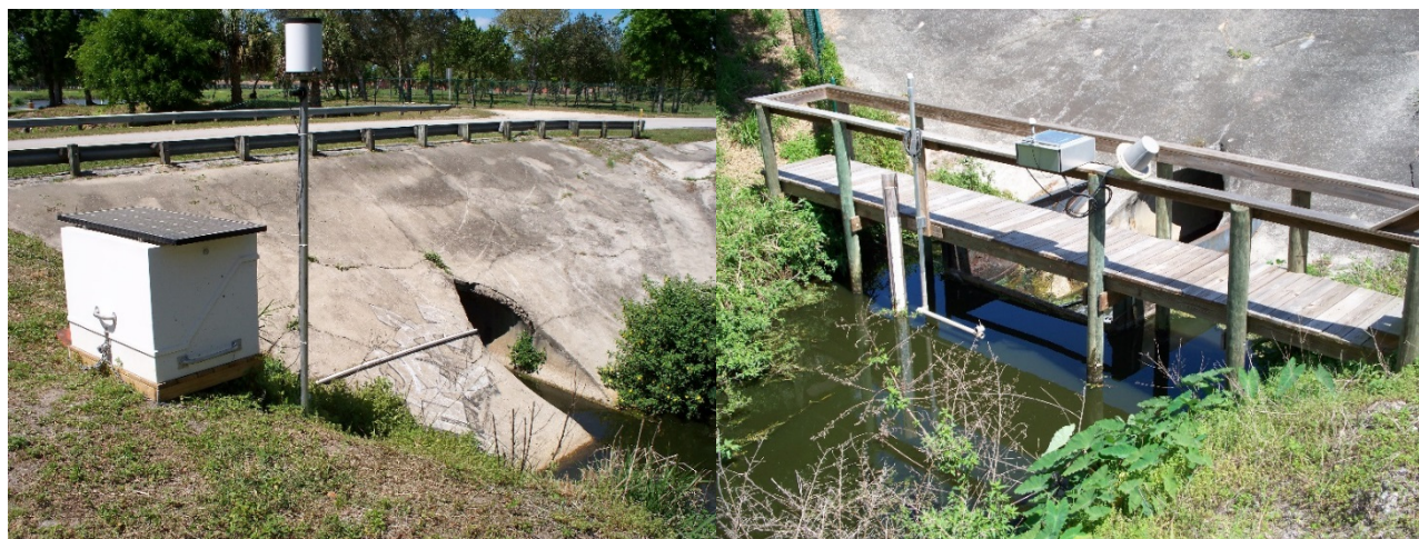
FIGURE 5: USGS MONITORING STATION ON PLAZA PARKWAY AT BRACCO RESERVOIR OUTFALL
