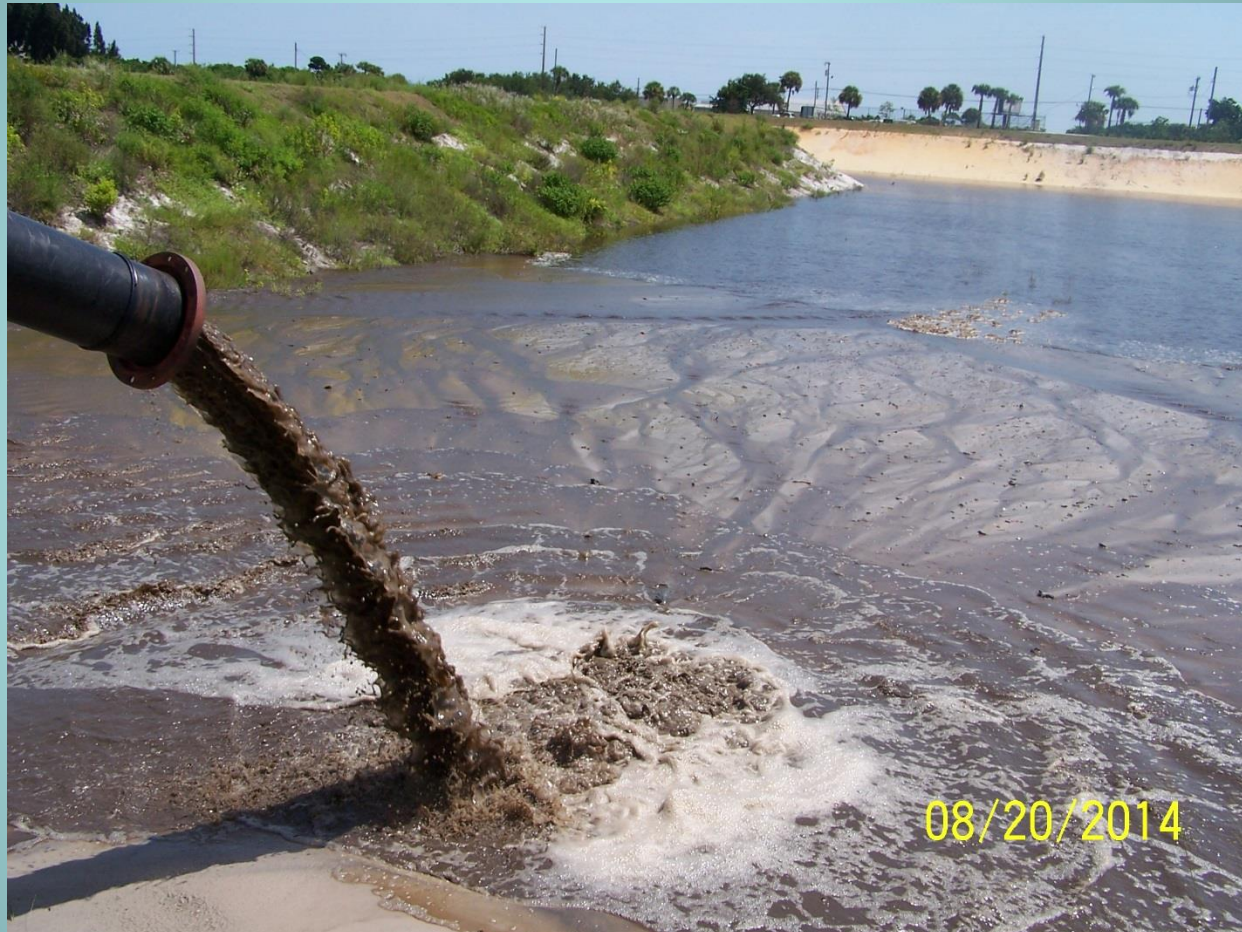
Dredge discharge pipe at Disposal Site
