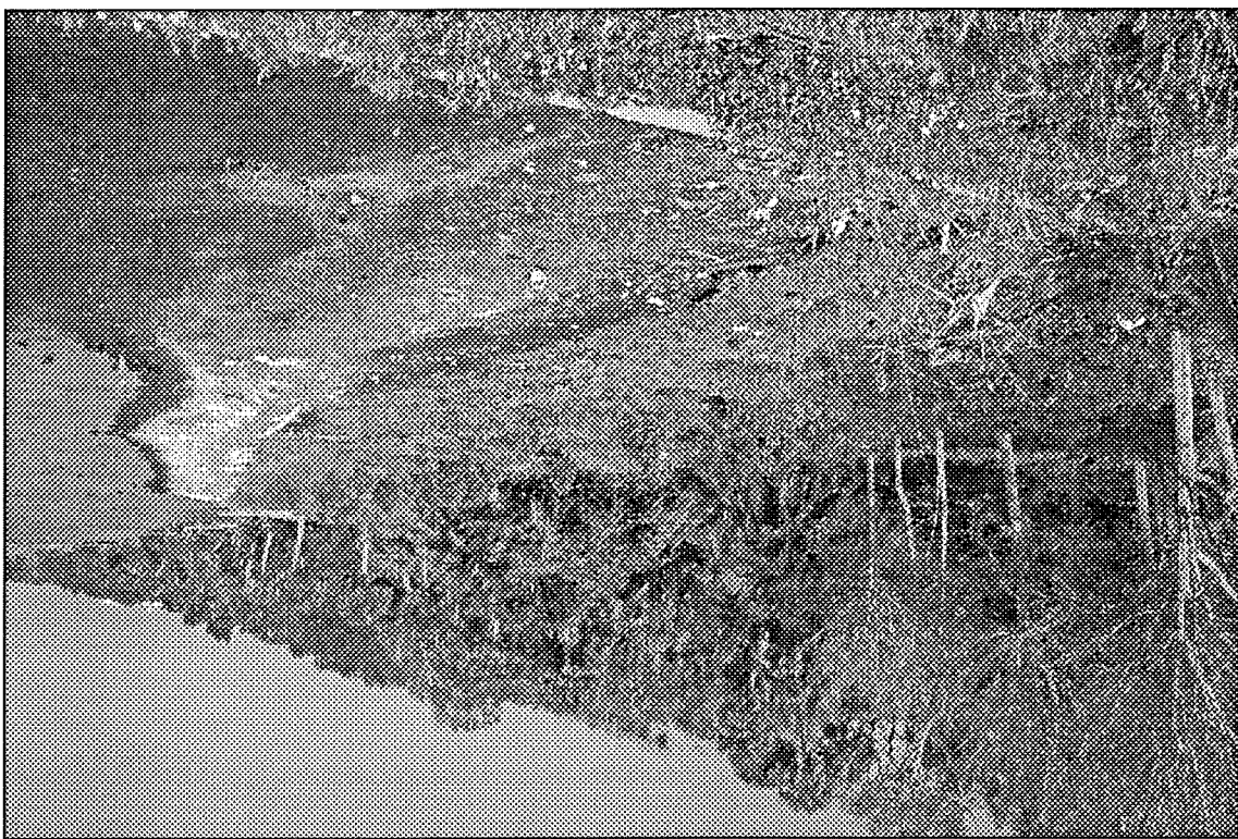
Photo 17 - View of erosion at West-Bound Melbourne (1-92) Causeway - Looking North
