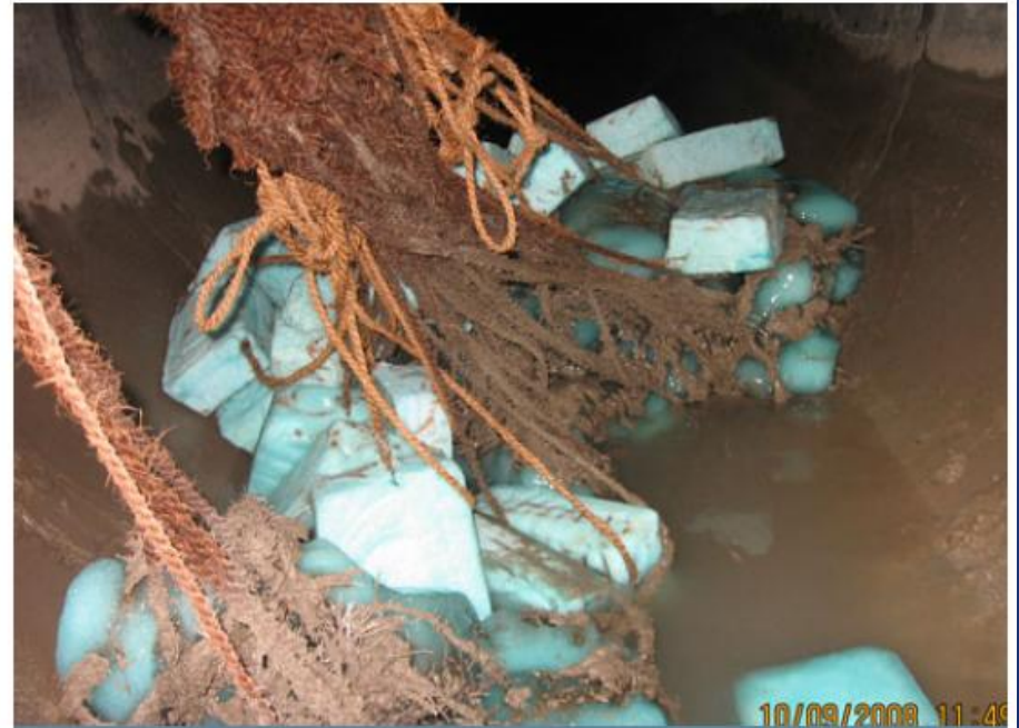
APS Floc Logs® in one of the 66" discharge pipes
