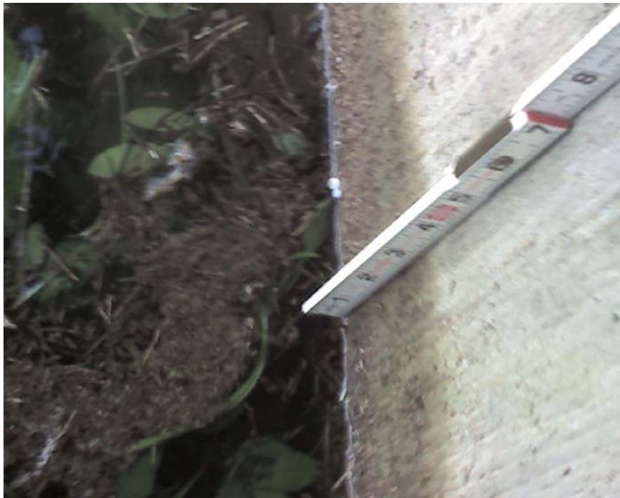
High water mark on weir wall. Photo taken August 20, 2008.
