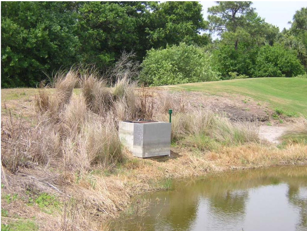
Water Control Structure WV-L29. Photos taken April 12, 2007.
