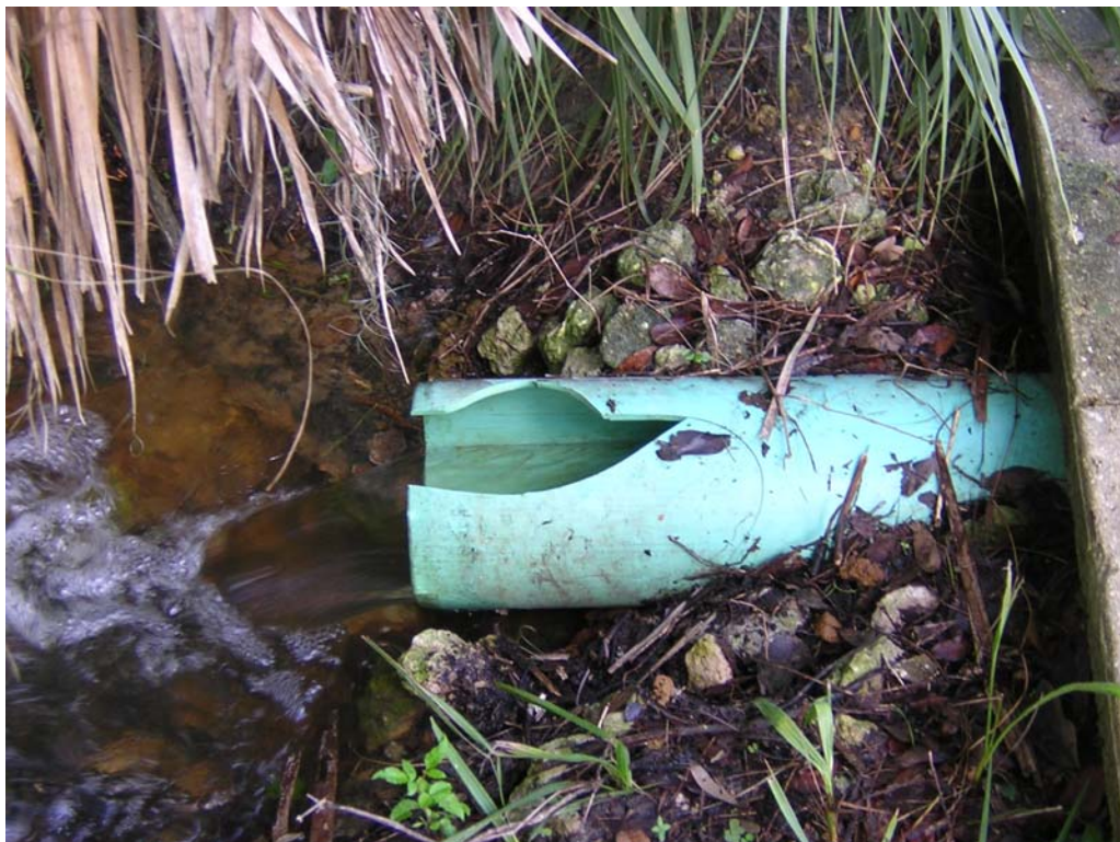
Discharge from L-12 structure. Photo taken July 17, 2008.
