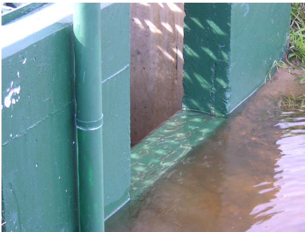
Water Control Structure SW-LA8 – unsubmerged flow. Photo taken July 17, 2008
