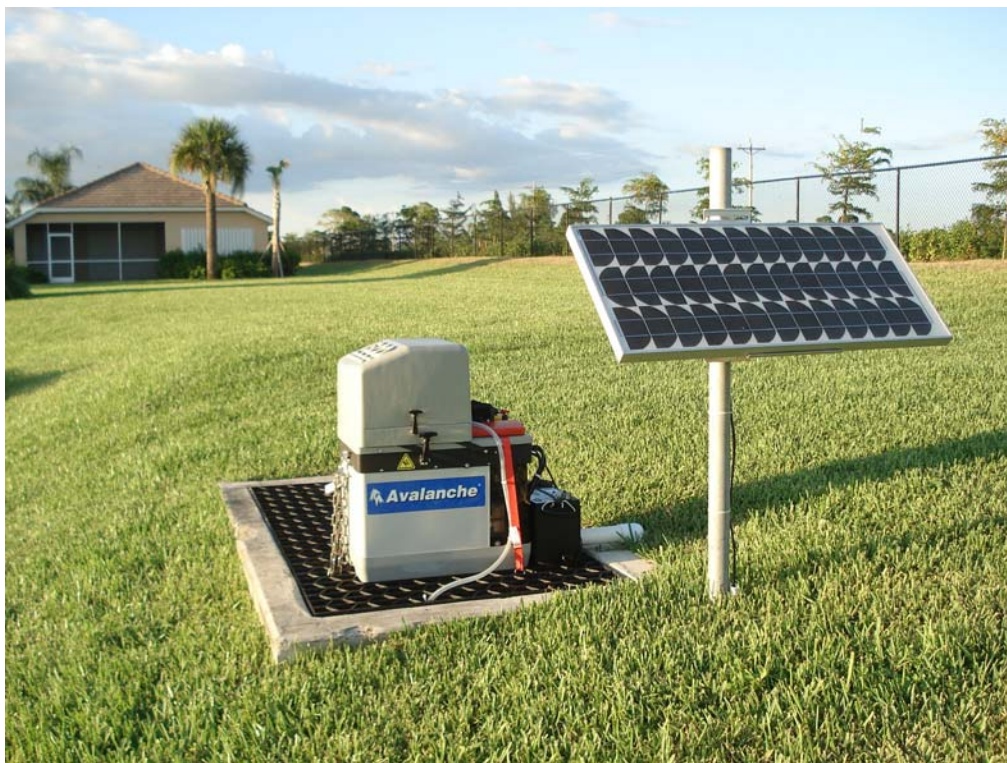
View north at WS-1 – September 13, 2008. Water quality monitoring. Solar panel at right.
