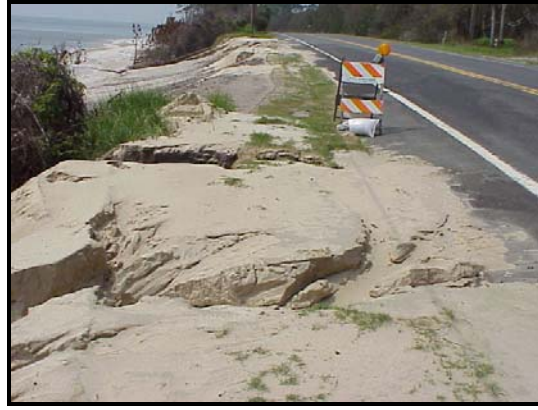
Sheet and gully erosion along shoulder, August 2005
