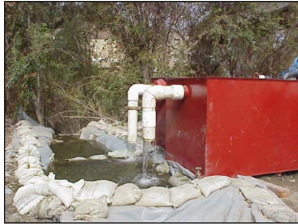
Dewatering Tank (Source: http://www.dot.ca.gov )
