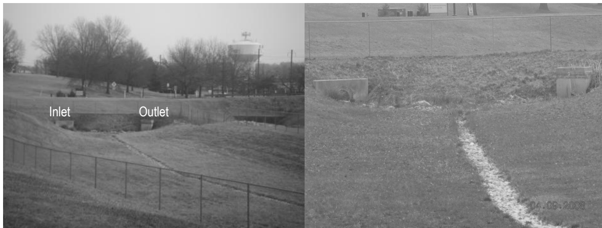
Figure 8-2. Poorly Designed Detention Pond (Distance and Close-Up View).
