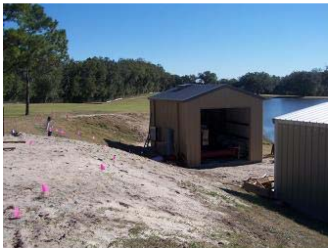
NEW RECLAIMED WATER PUMPING STATION WITH BUILDING
