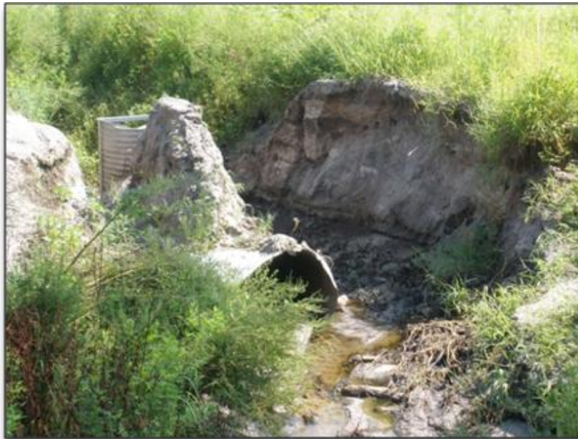
BLOWN-OUT CULVERT FROM SPRING STORMS
