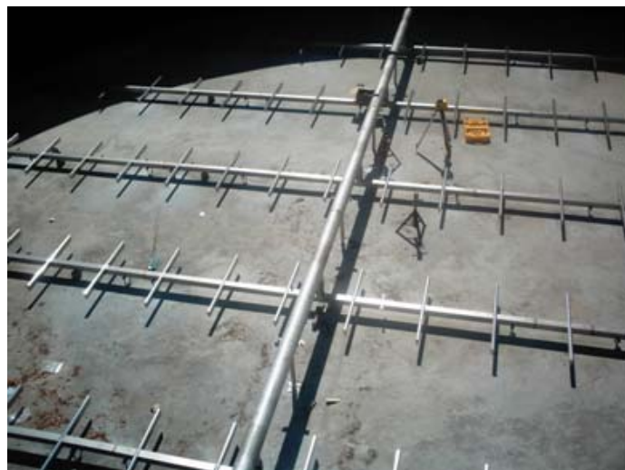
COARSE BUBBLE DIFFUSER ARRAY IN DIGESTER #2
