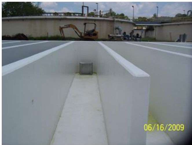
CHLORINE CONTACT CHAMBER CHANNEL WITH STAINLESS STEEL DIFFUSER BAFFLE AT INFLUENT
