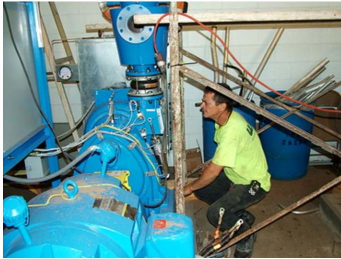
INSTALLED MORE EFFICIENT BLOWERS
