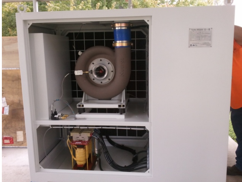
ASH STREET WWTF NEUROS TURBINE BLOWERS
