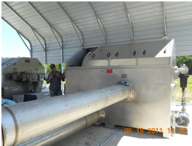
TERTIARY FILTER #2 AT THE ASH STREET WWTF
