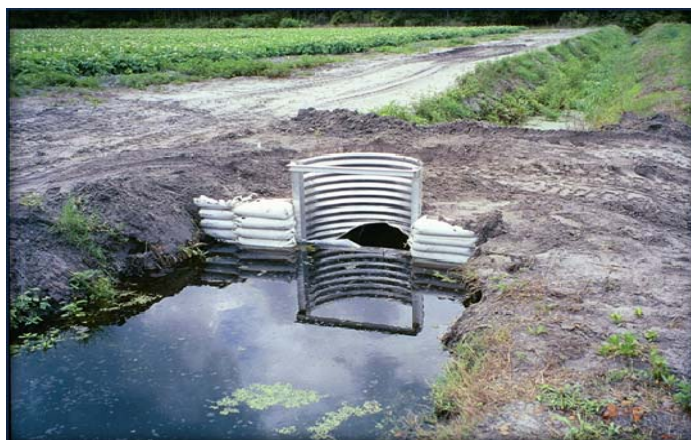
FIGURE 42: WATER CONTROL STRUCTURE TO MANAGE DITCH LEVELS AND SEEP IRRIGATION
