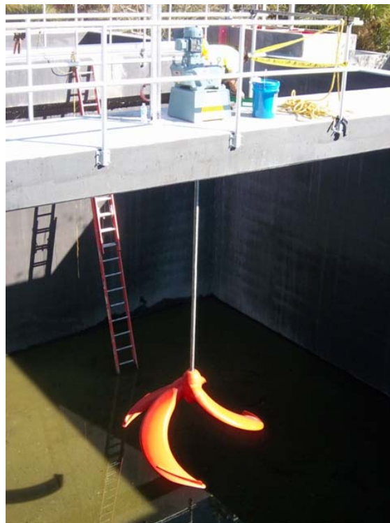
NEW MIXERS INSTALLED THE ANOXIC ZONES
