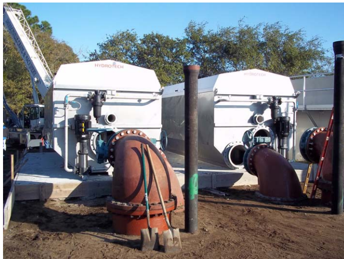
EFFLUENT FILTERS INSTALLED AT WWTP #1
