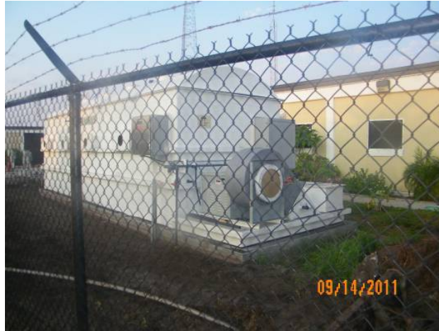
FIGURE 11: JACKSONVILLE BEACH WWTP NEW ODOR CONTROL EQUIPMENT
