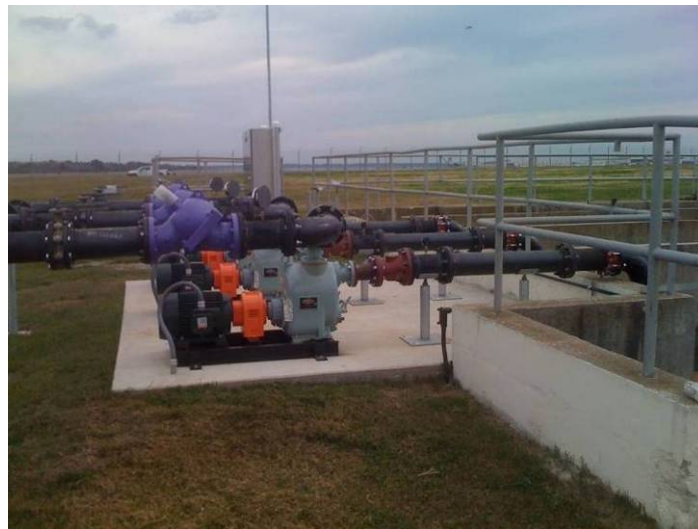
FIGURE 22: NEW REUSE PUMPS FOR PHASE 1 EXPANSION AT NAS JACKSONVILLE
