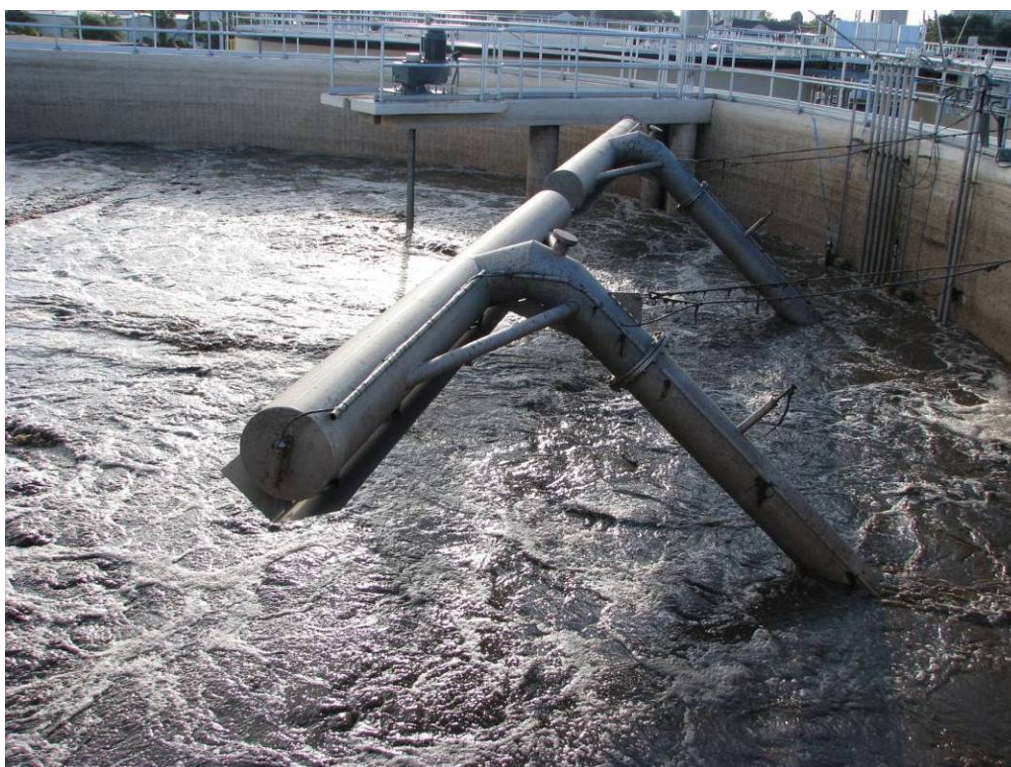
NEW DECANT MECHANISM ON THE SEQUENCING BATCH REACTOR TANK
