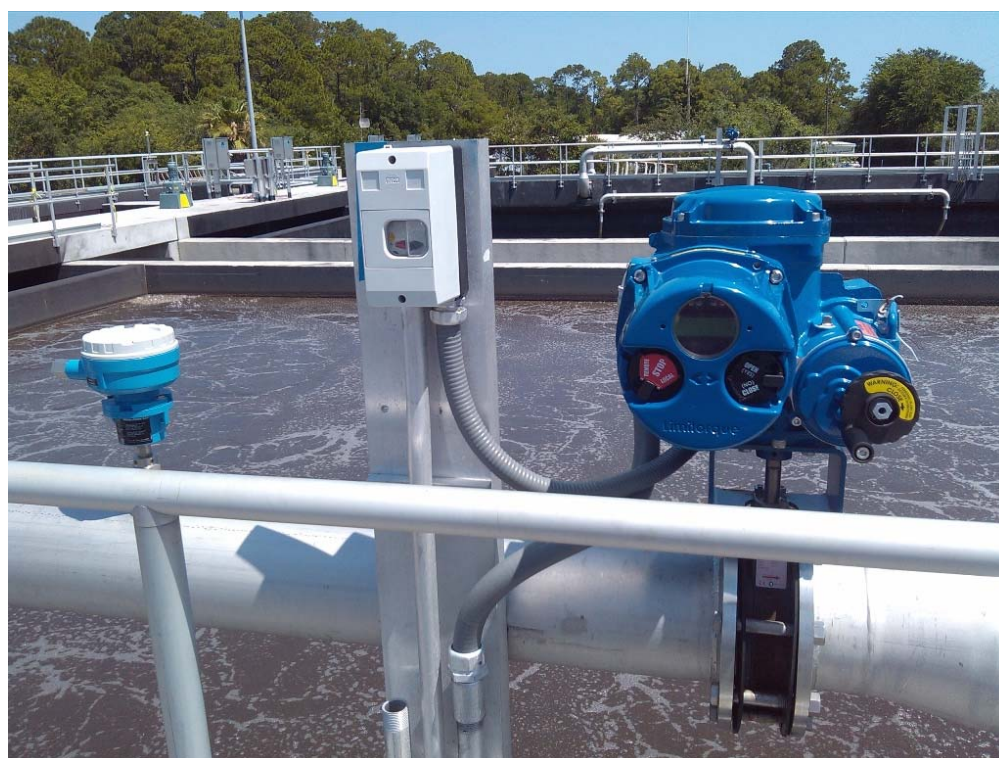
AUTOMATED VALVES CONTROL AIR FLOW TO AERATION BASINS
