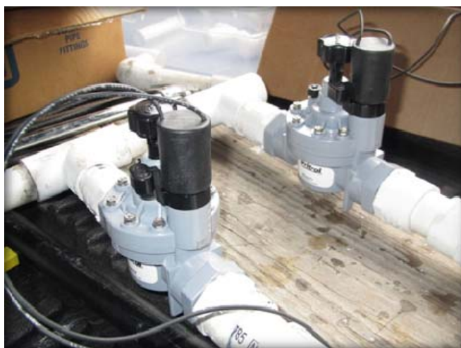
MANIFOLDS WITH VALVES ATTACHED TO END OF EACH DRIP TAPE LINE TO REGULATE/DIRECT FLOW OF WATER
