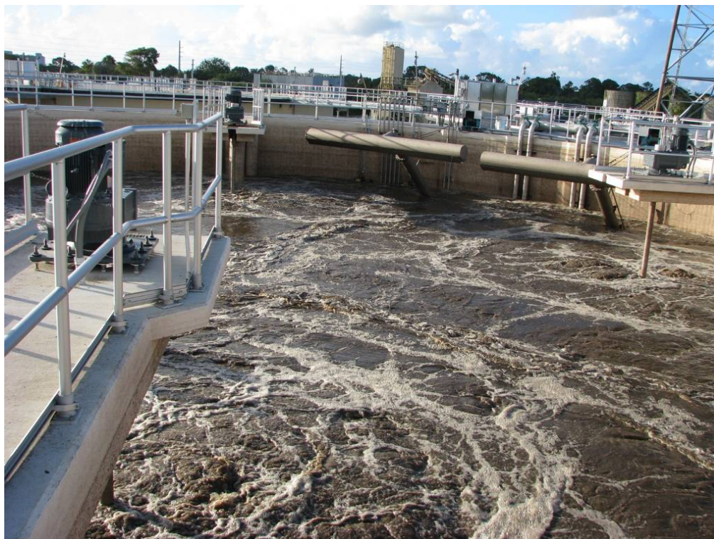
NEW SEQUENCING BATCH REACTOR TANK
