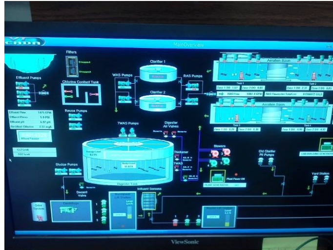
NEW SYSTEM ALLOWS OPERATORS TO MONITOR AND CONTROL ALL PLANT FUNCTIONS
