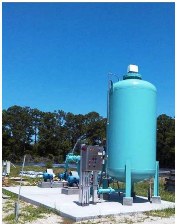
ON-SITE REUSE SYSTEM INSTALLED FOR WATER CONSERVATION
