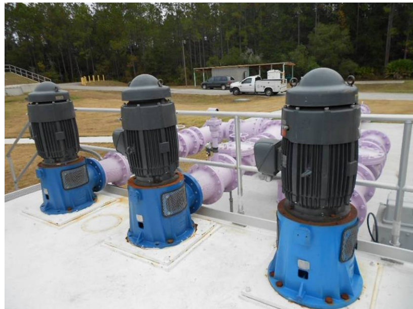
FIGURE 4: CITY OF PALATKA WWTP NEW AERATION SYSTEM
