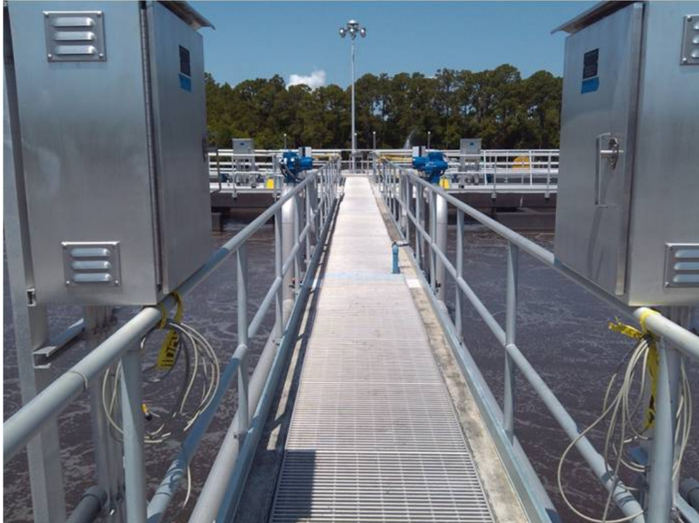
REMOTE MONITORS MEASURE DISSOLVED OXYGEN TO DETERMINE BLOWER AND VALVE CONFIGURATION
