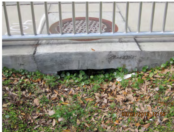
FIGURE 12: STORMWATER INLET IN NEED OF MAINTENANCE
