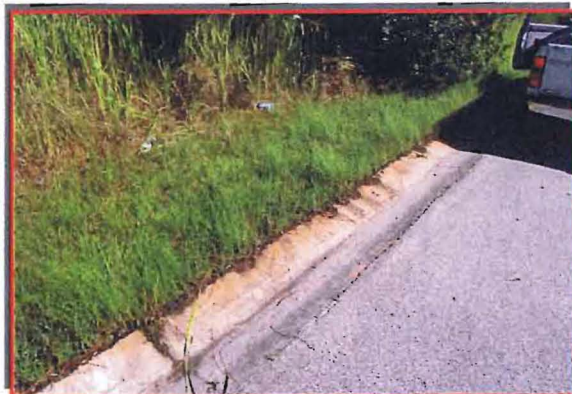
PHOTO 3: VIEW OF SEEPAGE ALONG CURBLANE ALONG KANE COURT NEAR WETLAND.
