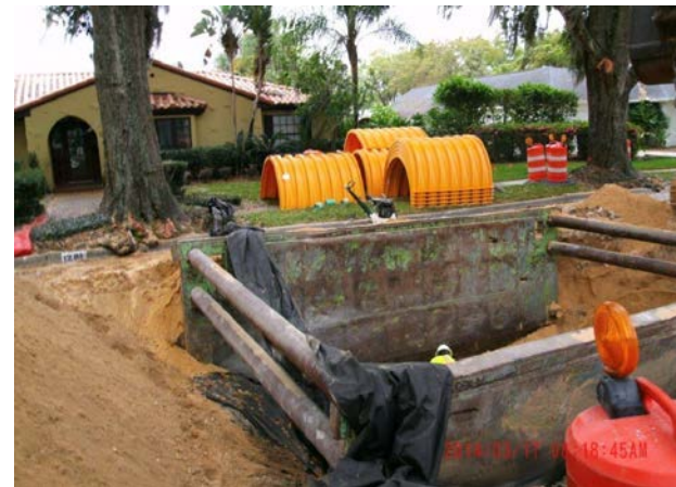
City of Winter Park North Exfiltration Treatment Project
