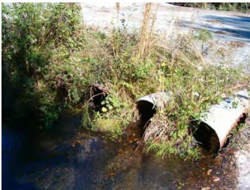
Figure 7 – Bleeddown Pipes from Pond A-2
