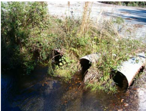
Figure 7 – Bleeddown Pipes from Pond A-2
