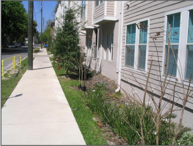
Figure 3.11. Disconnected roof gutters at the Oxford Terrace Apartments
