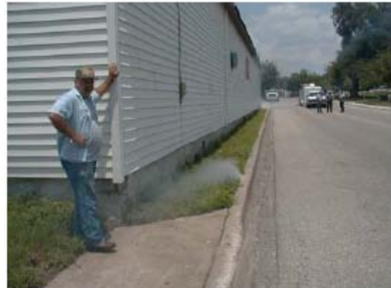
Broken Service Lateral
