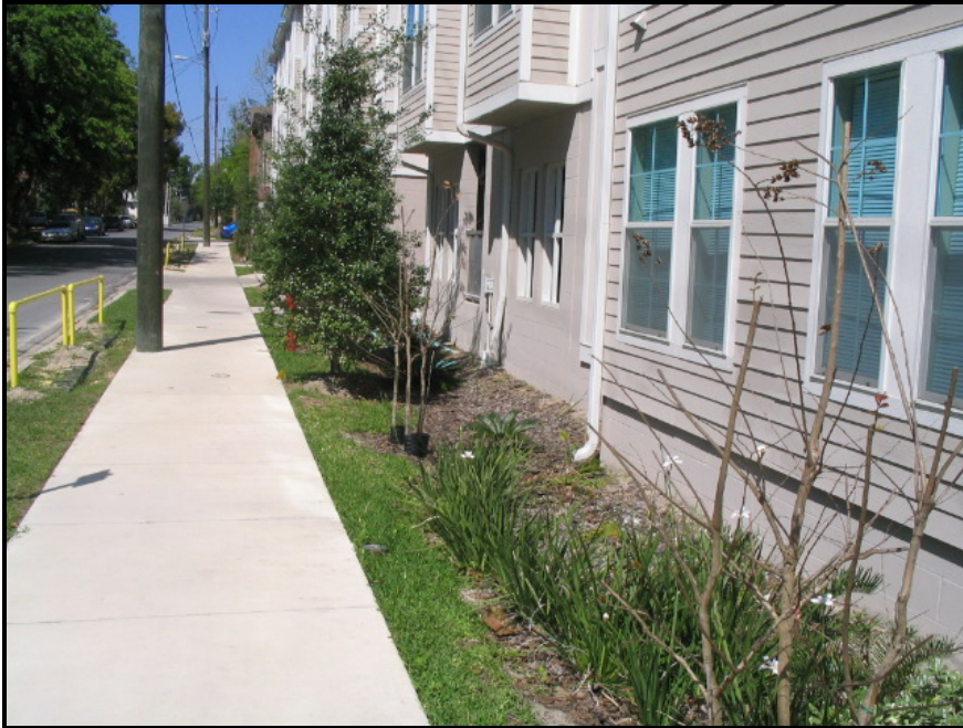
Figure 36. Disconnected roof gutters at the Oxford Terrace Apartments
