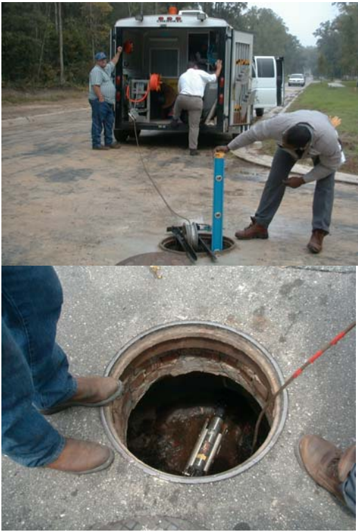
Figure 29. GRU Closed-Circuit TV Inspection Unit
