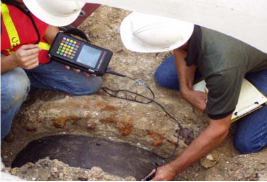
Figure 35. GRU Engineers and Crews Performing Pipe Wall Thickness Testing
