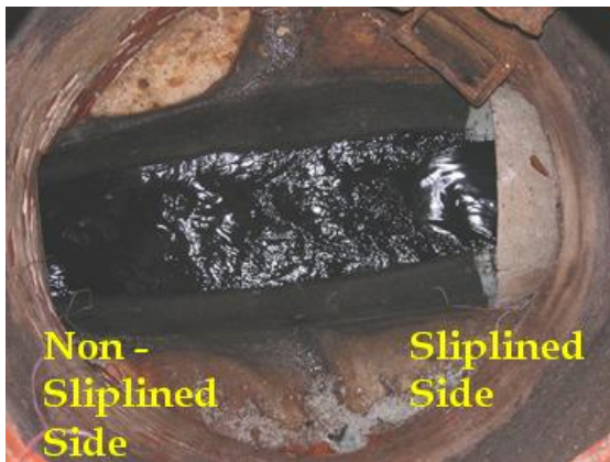
Figure 33. Pictures of a Sliplined Pipe near Hogtown Creek
