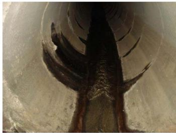
A) View looking downstream of groundwater seepage in cracks in the Gutierrez Stormdrain Line at monitoring location 11
