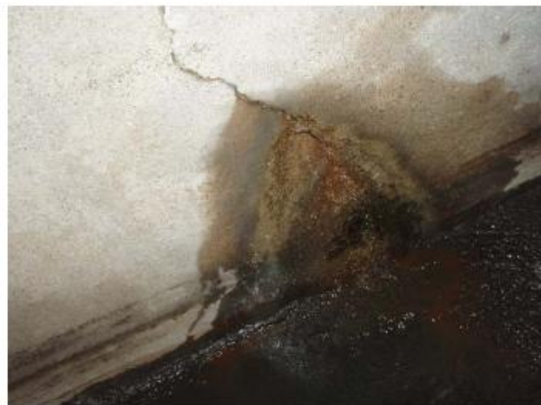
B) Drop inlet wall at southern corner of Ortega Park with groundwater trickling into crack in the inlet wall.
