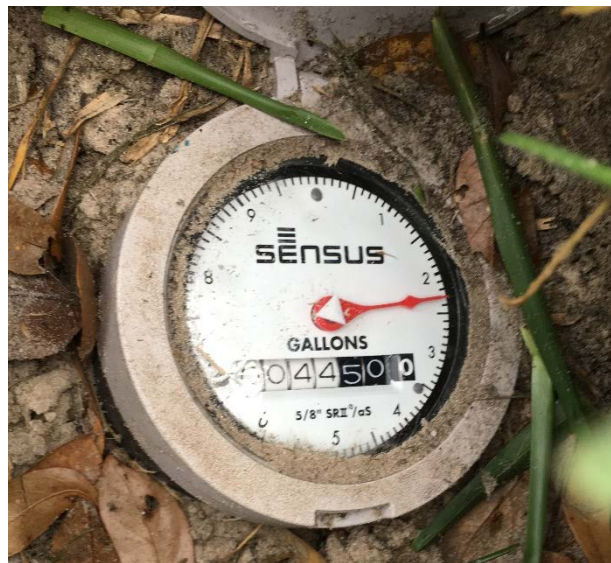
Figure 12 Flow gauge (located downstream of septic tank, prior to flow into passive system.
