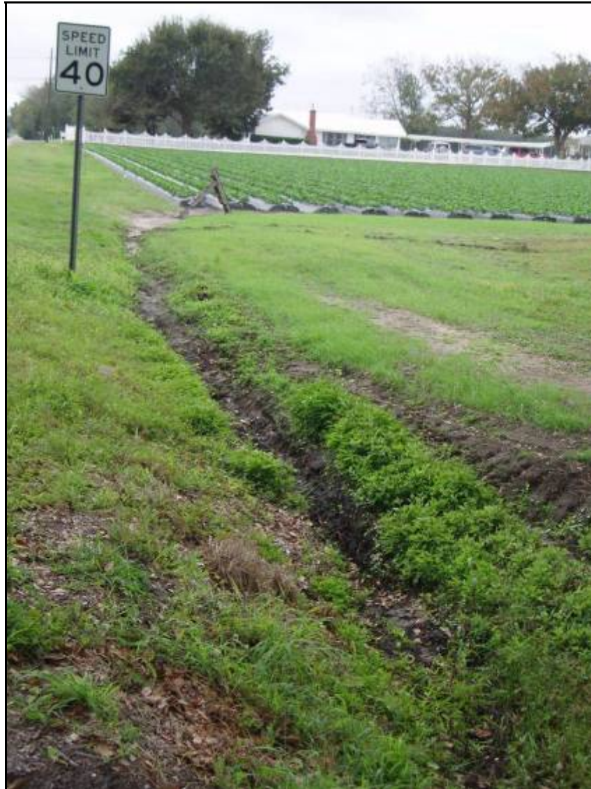
Figure 10. Erosion from a strawberry field toward the cross drain in Figure 8. While the photo depicts a discrete instance, erosion from agricultural lands was commonly observed during the Walk. Erosion causes sedimentation in ditches and creeks, which may create favorable conditions for fecal coliform bacteria.
