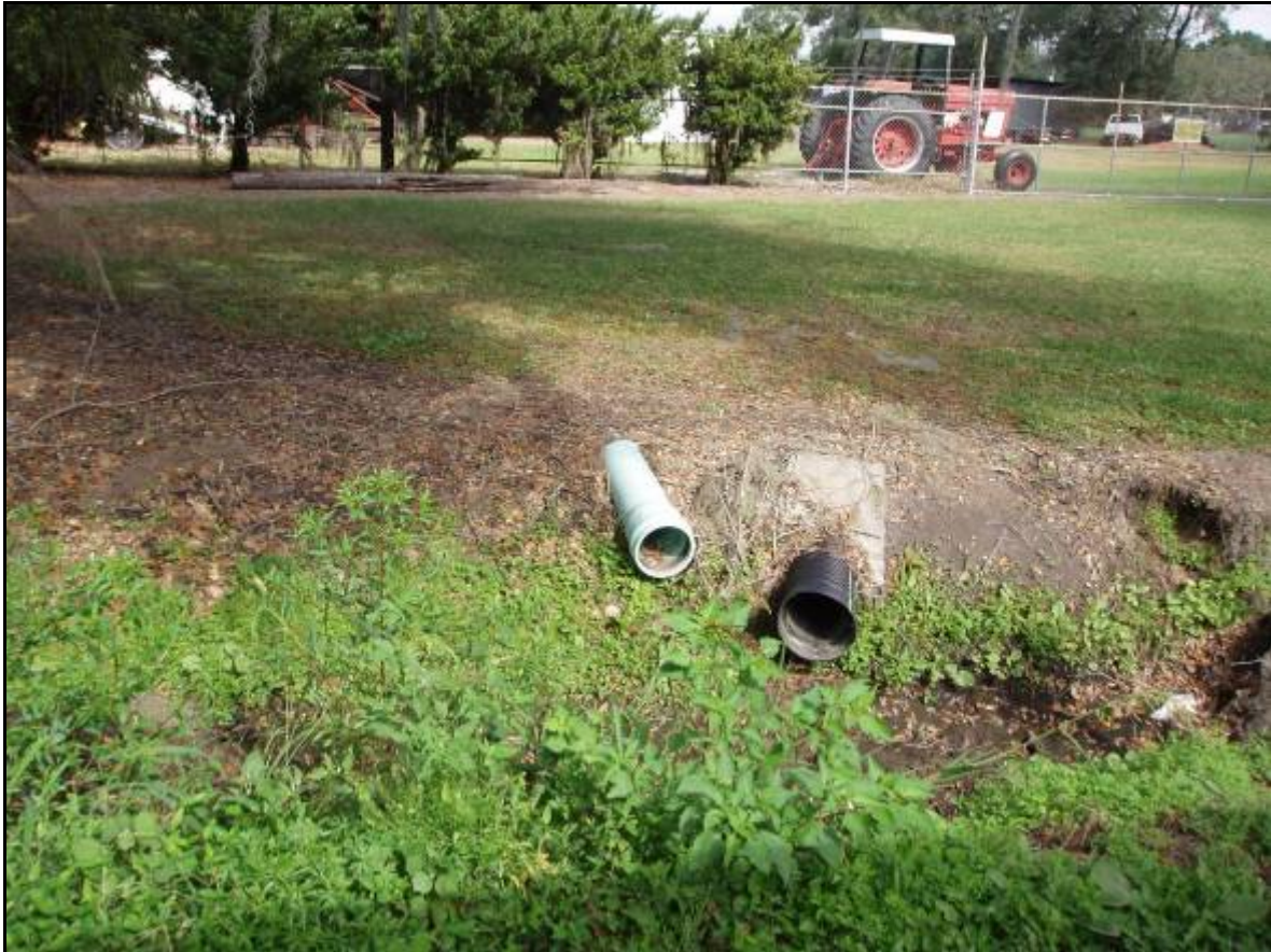
Figure 23. Potential illicit connections on Caruthers Ave. near Sydney Rd. Pipes protrude from the parcel into the roadside ditch. Referred to EPC for enforcement.
