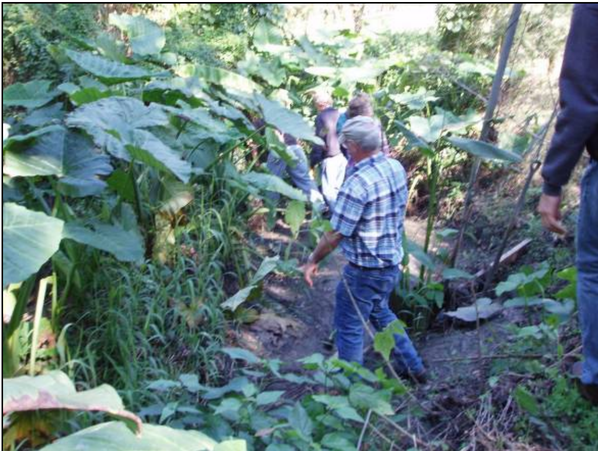
Figure 50. Likewise, the ditch/tributary, which runs behind Starlite MHP to Turkey Creek, is similarly overgrown and harboring trash and excess sediment.
