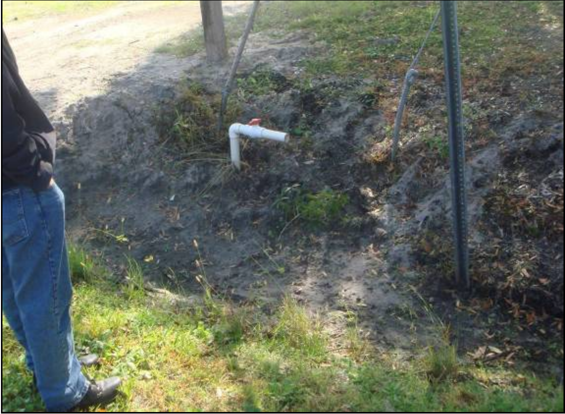
Figure 24. Potential illicit connection on Caruthers Ave near Turkey Creek crossing. Pipe is adjacent to a strawberry field and enters the roadside ditch.
