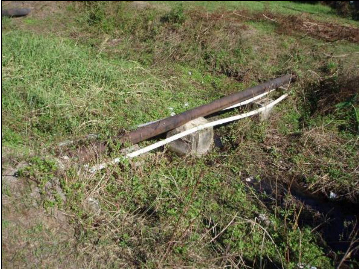
Figure 31. Pipes crossing a ditch in Starlite MHP. These pipes appear to be a part of the onsite wastewater treatment facility. No leaks were witnessed. However, the mobile home park is largely abandoned, in disrepair, and has a history of deficient wastewater treatment plant.
