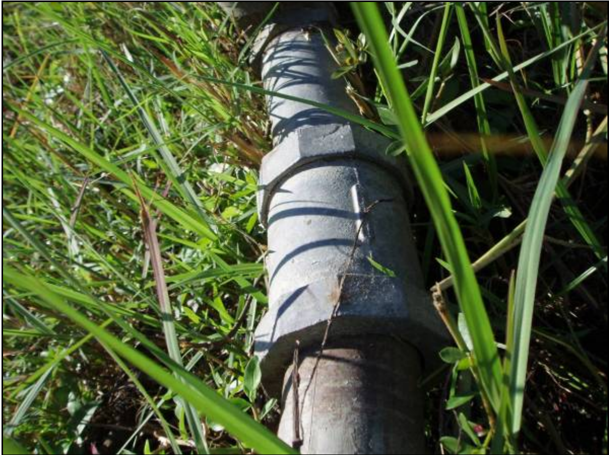
Figure 33. Close up of pipe in Figure 32, which shows the disconnection at the pipefitting.
