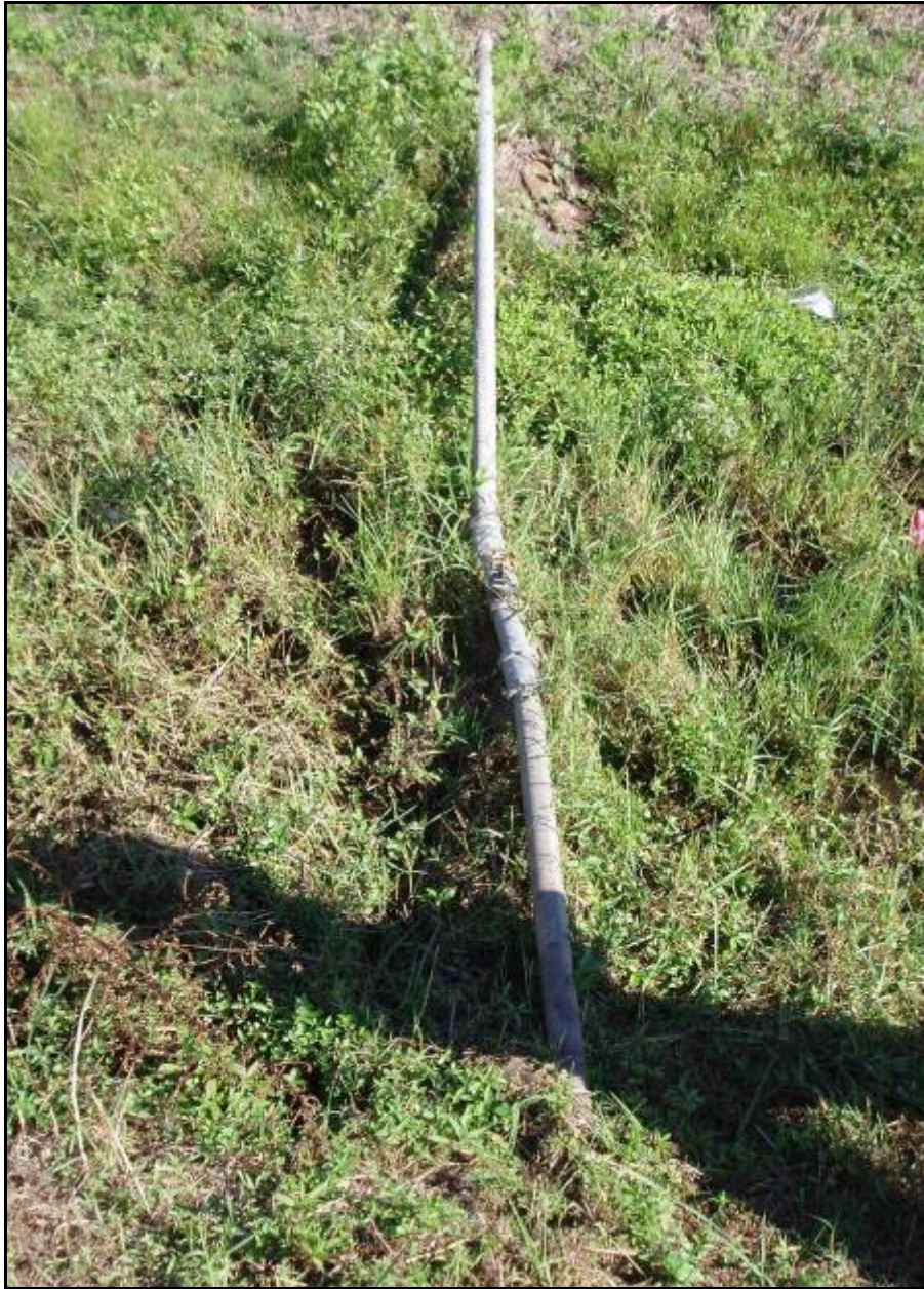
Figure 32. Another unknown pipe crossing a ditch in Starlite MHP. This pipe is not connected properly with a high likelihood of leaking should effluent or other liquids be transported. No leaks witnessed while onsite.
