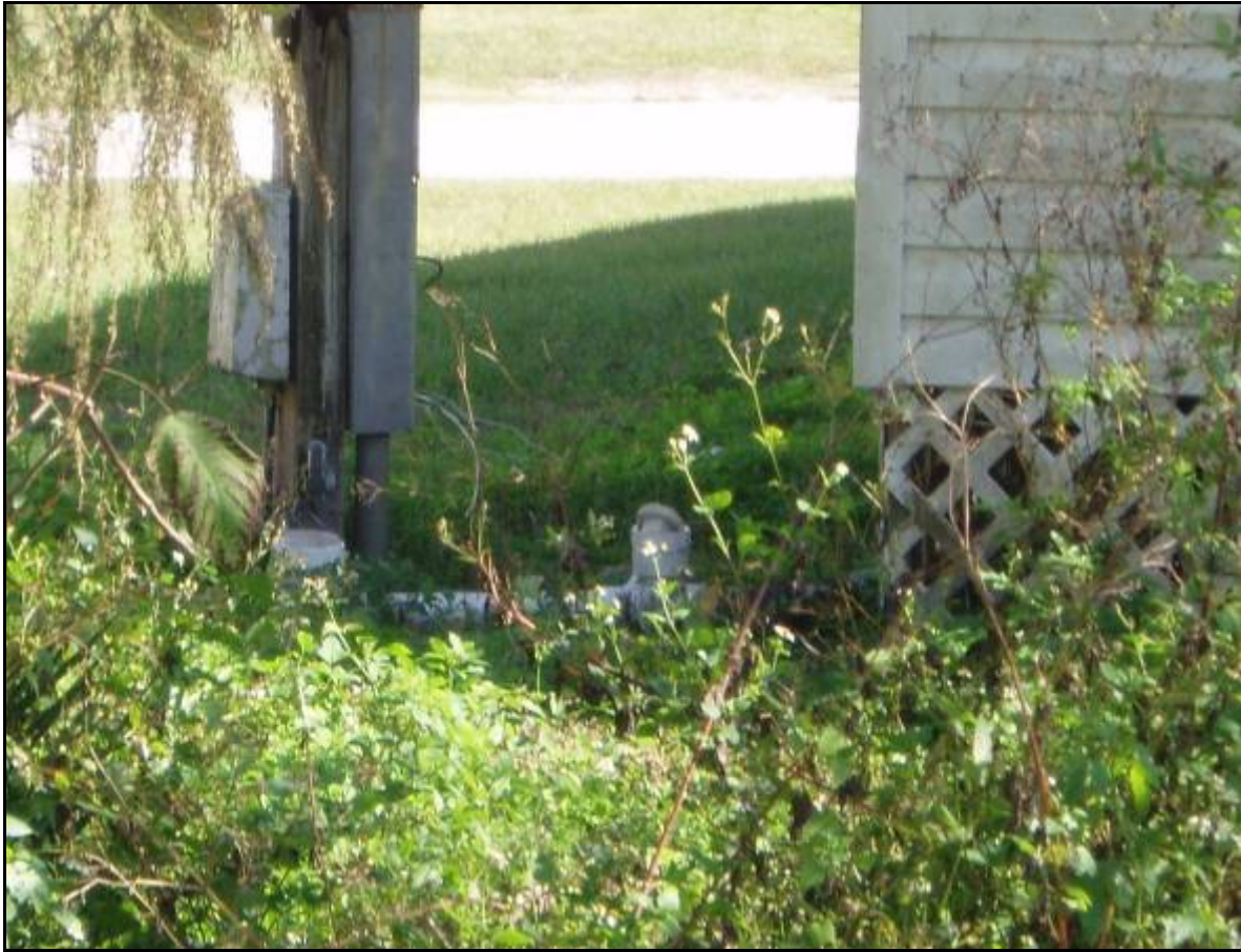
Figure 35. Several wastewater cleanouts were uncapped throughout Starlite MHP. While many of the homes appeared abandoned, i.e. system not in use, there is potential for illegal inhabitation, and cleanouts are often in close proximity to stormwater conveyances.
