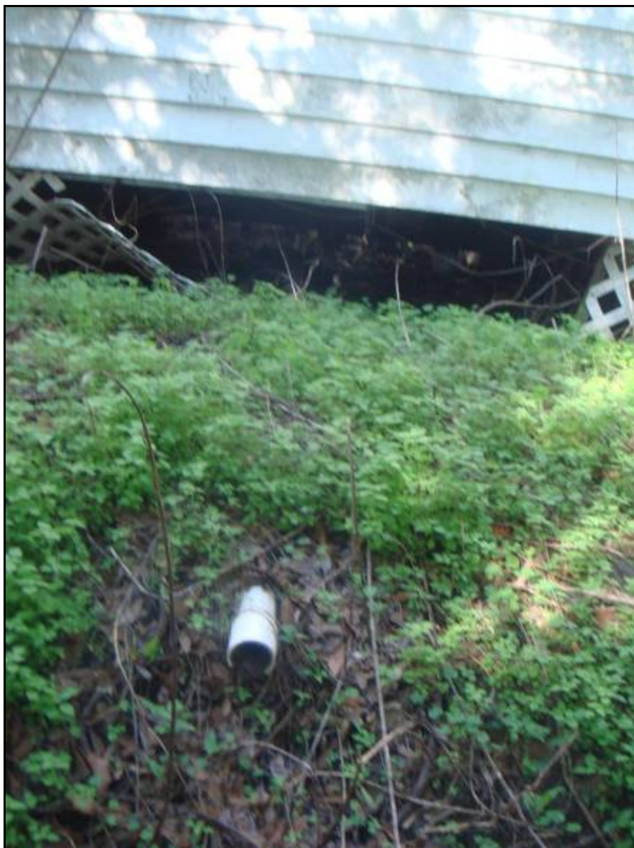
Figure 37. Another unknown pipe extending from underneath a mobile home at Starlite MHP into a stormwater conveyance.
