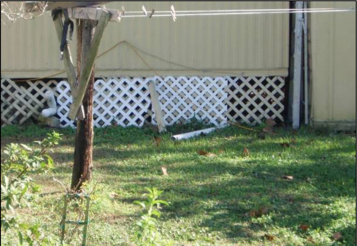
Figure 36. Unknown pipe extending from underneath a mobile home at Starlite MHP. Appearance is consistent with the discharge of washing machine grey water.
