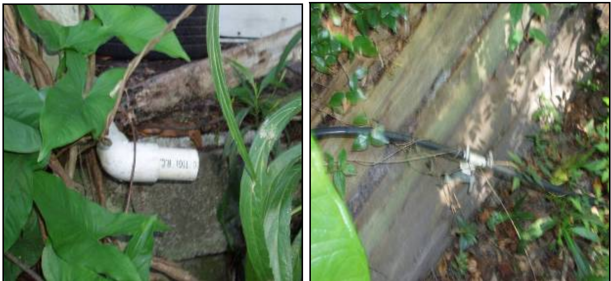
Figure 51. Potential illicit connections to ditch/tributary along the northern edge of Starlite MHP. PIC is located near the northern terminus of Marge Owens Rd.
