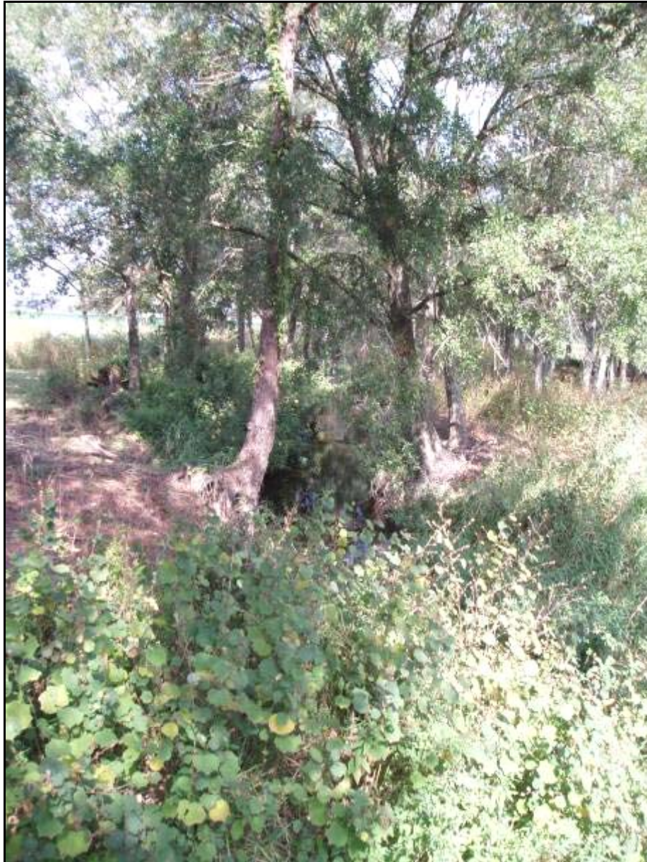
Figure 25. Turkey Creek at Caruthers Ave. Some overgrowth of invasive vegetation.
