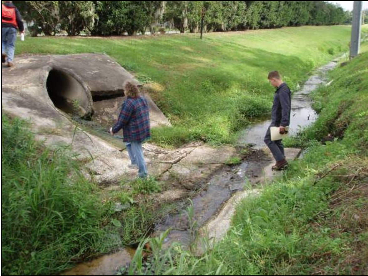
Figure 16. Outfall from Walden Lakes community located on Trapnell Rd west of Timberlane Dr. The outfall drains the southern half of Walden Lakes subdivision. Significant erosion was present.
