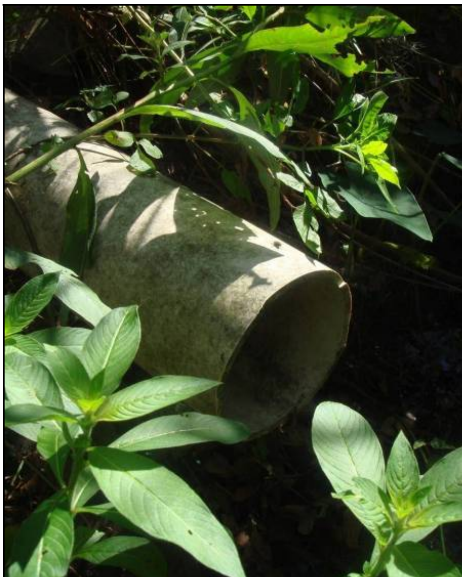
Figure 53. Potential illicit connection into tributary at Jerry Smith Rd between Trapnell & Sydney. The trajectory of the pipe appears to lead to a mounded septic system. No discharge witnessed while onsite. Referred to DOH for nuisance complaint investigation.
