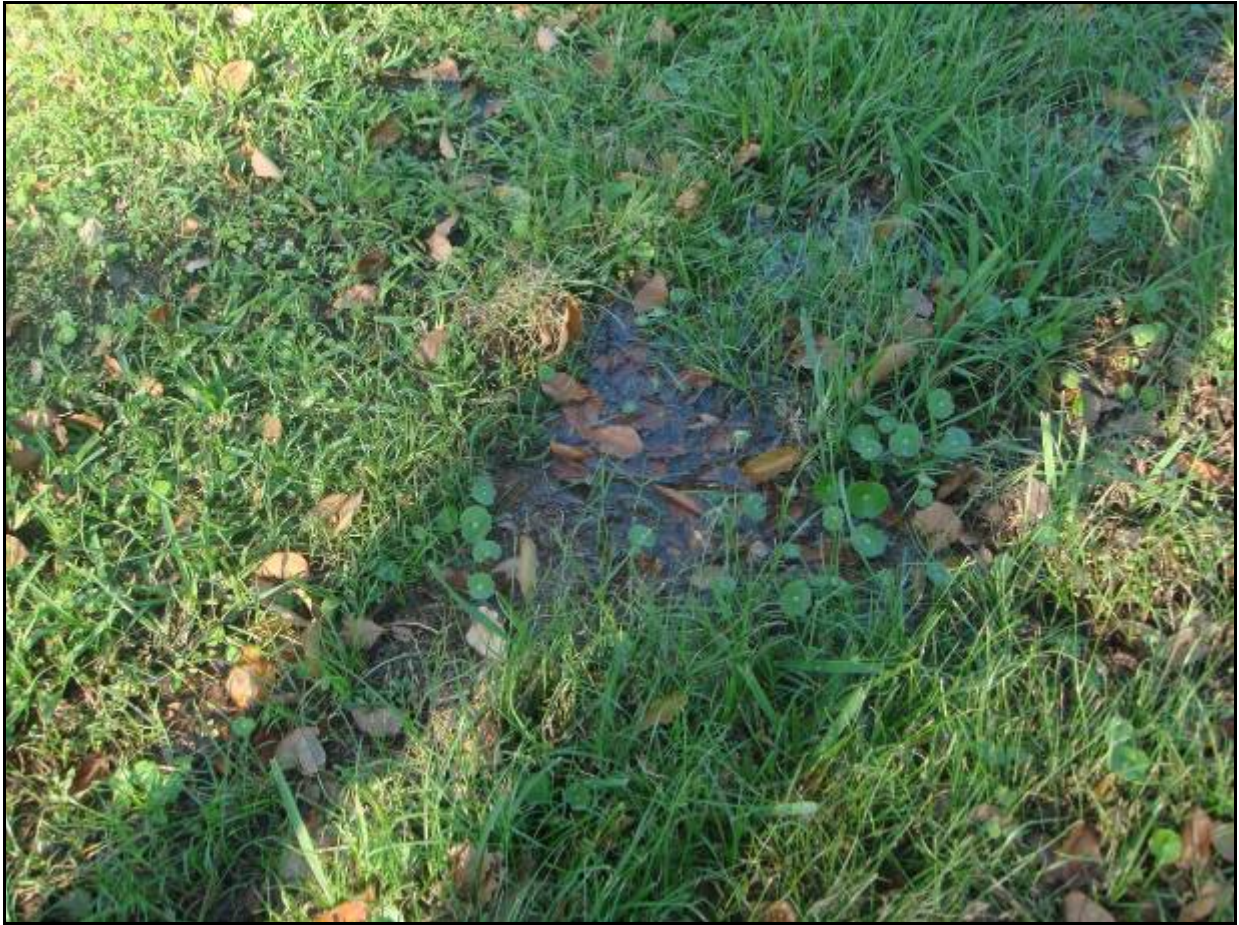
Figure 59. Septic drain field at Crawford 3B's Mobile Home Park is super-saturated and ponding. The effluent was observed adjacent to the Turkey Creek tributary. EPC notified the owner of the concern during the Walk and directed to resolve the violation. Re-inspection should confirm proper functionality.
