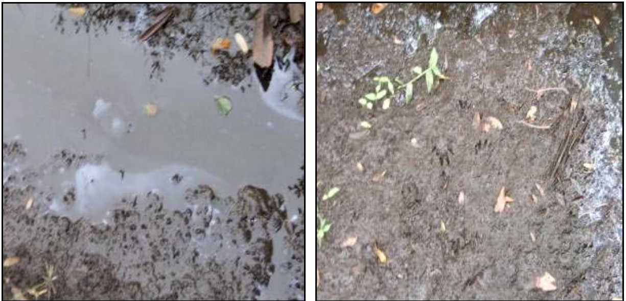
Figure 9. Close up of oily sheen and raccoon tracks at cross drain shown in Figure 8. Oily sheen appeared to be a natural condition attributed to sediment characteristics.
