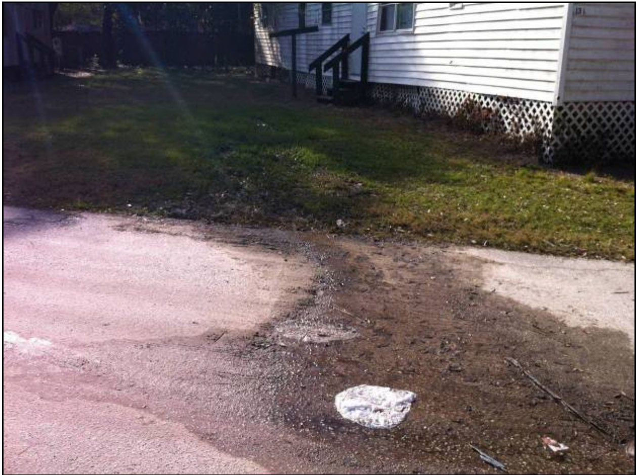
Figure 39. Follow up inspection on 01/24/12 showed saturation in Figure 38 persists and has increased considerably. Standing water present and continues down the street. The water contained no detectable odor or discoloration. Referred to EPC for investigation.
