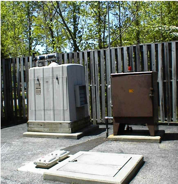
Figure 1C: Typical Large Pump Station
