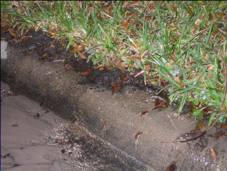
Broken Line Discharges Into Gutter
