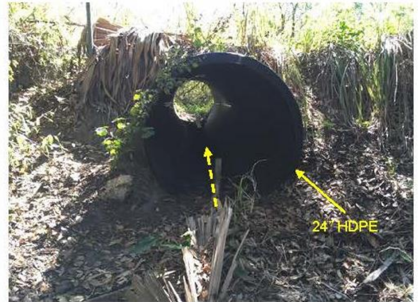
Outfall pipe through earthen berm
