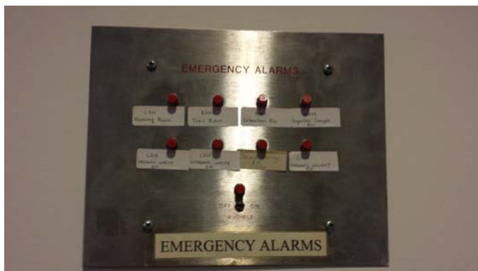
Figure 5.4.1 Emergency Alarms Panel
