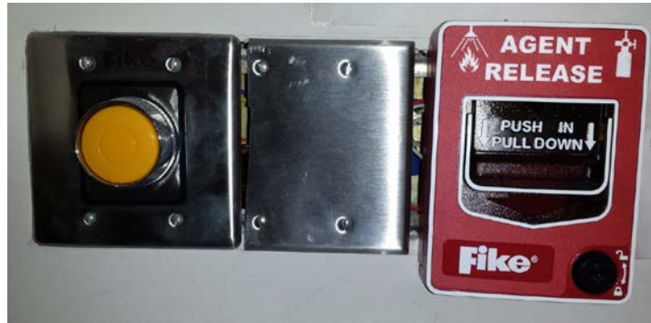
Figure 2.3.1 Halon Release Panel
