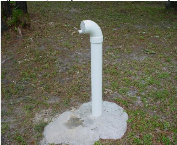
Figure 50. No, it is a faucet connected to a municipal water supply at a county park.
