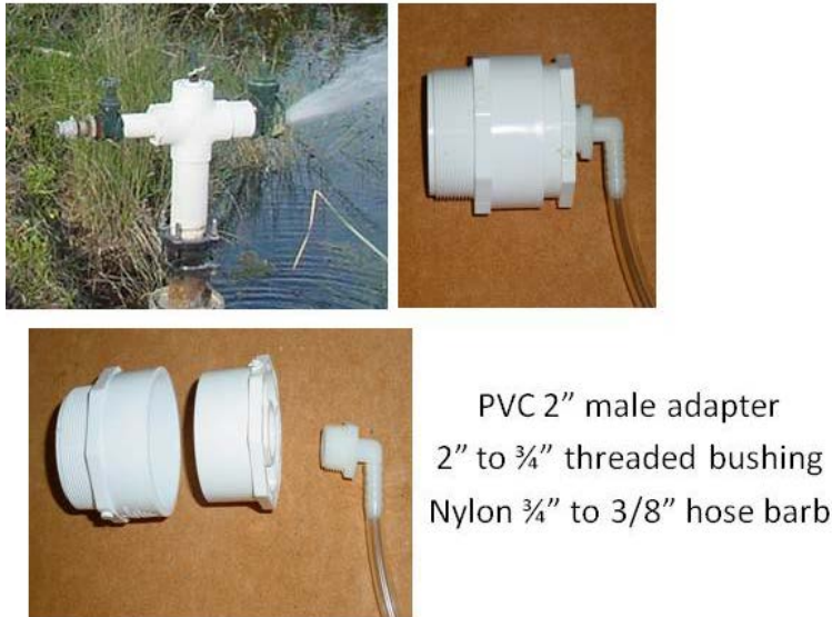
Figure 37. Example of a well that needs a PVC adapter. It is important to note specific requirements, such as the size of needed adapters, during field recon.
