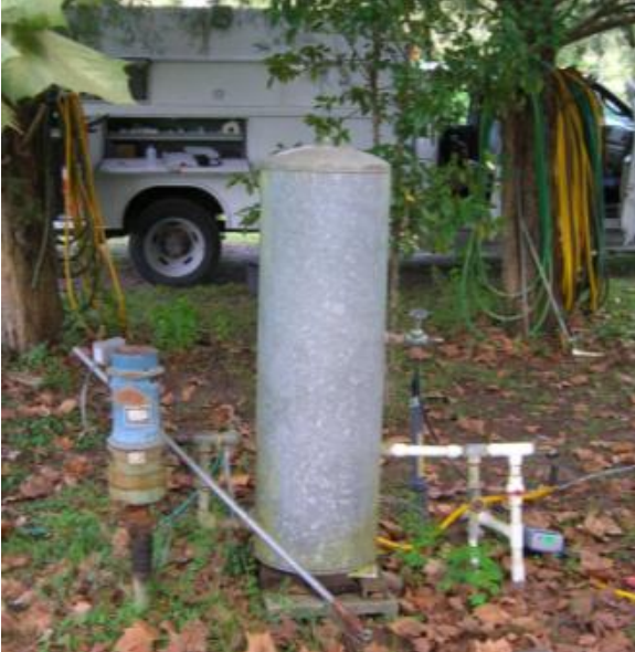
Figure 45. Private well with tank, but no softener or filter.
