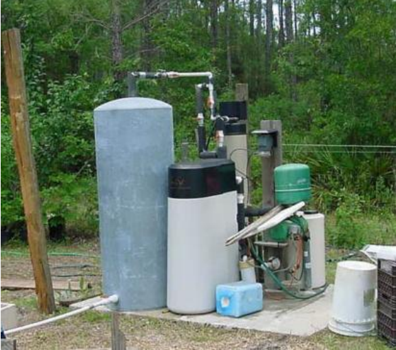
Figure 44. Private well with tank, softener, and filter.
