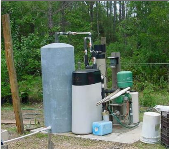
Figure 43. Private well with tank, softener, and filter.
