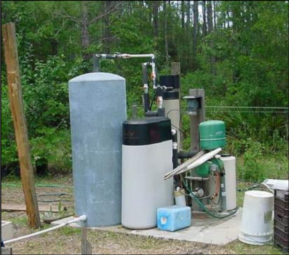
Figure 43. Private well with tank, softener, and filter.
