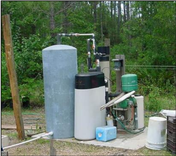
Figure 43. Private well with tank, softener, and filter.
