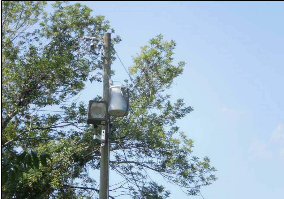
Photograph 9 – View of pole-mounted transformer located on the southern portion of the Property.
