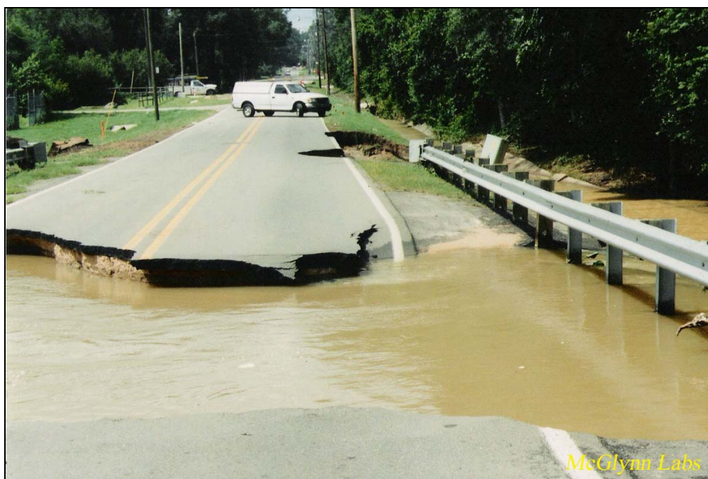
Figure 5.1.10: Stormwater laden with pollutants washes out Weems Road as Weems Pond, a stormwater treatment facility is overwhelmed, June 2001
