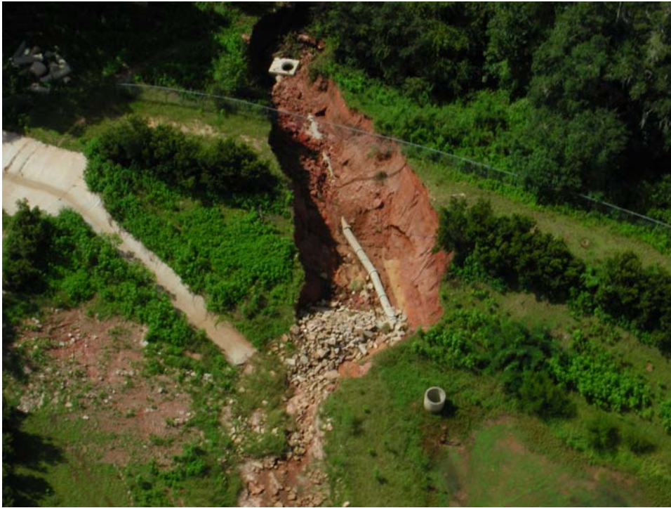
Figure 5.1.2.3: 2002 aerial photograph; The berm on the holding pond north of Lake Piney Z failed after Tropical Storm Berl.
