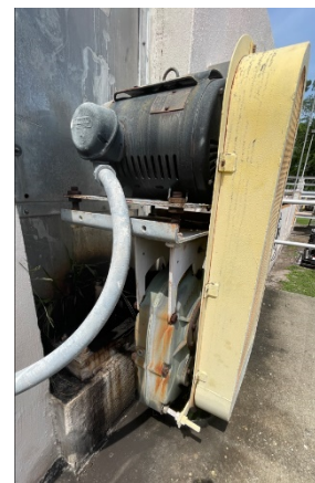
AERATOR SHAFT, MOTOR AND DRIVE
