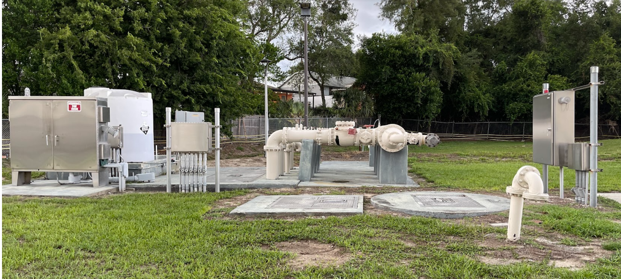
INTERMEDIATE PUMP STATION
