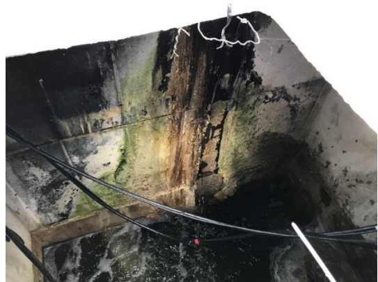
DAMAGE OF CONCRETE IN INTERIOR OF INTERMEDIATE PUMP STATION
