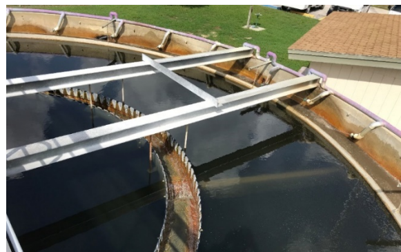
RUST AND CORROSION ON CLARIFIER 2
