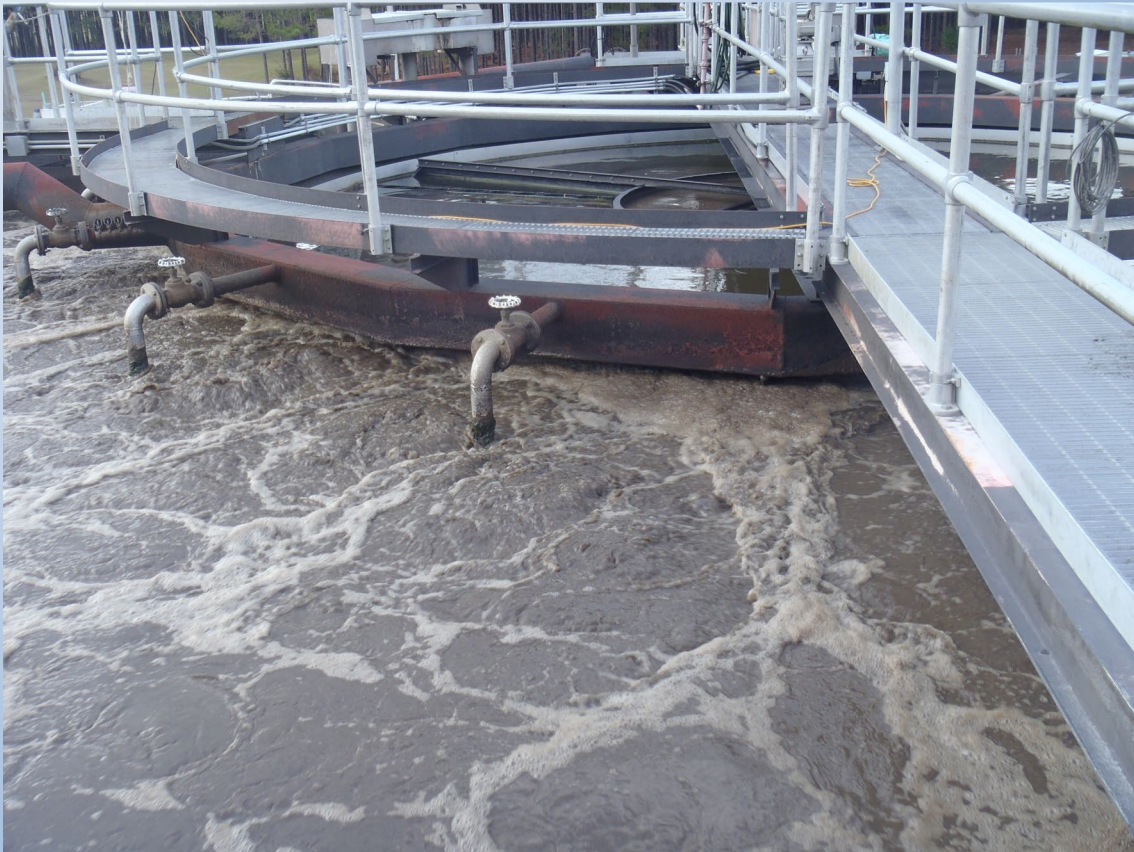
The City of High Springs aeration basin
