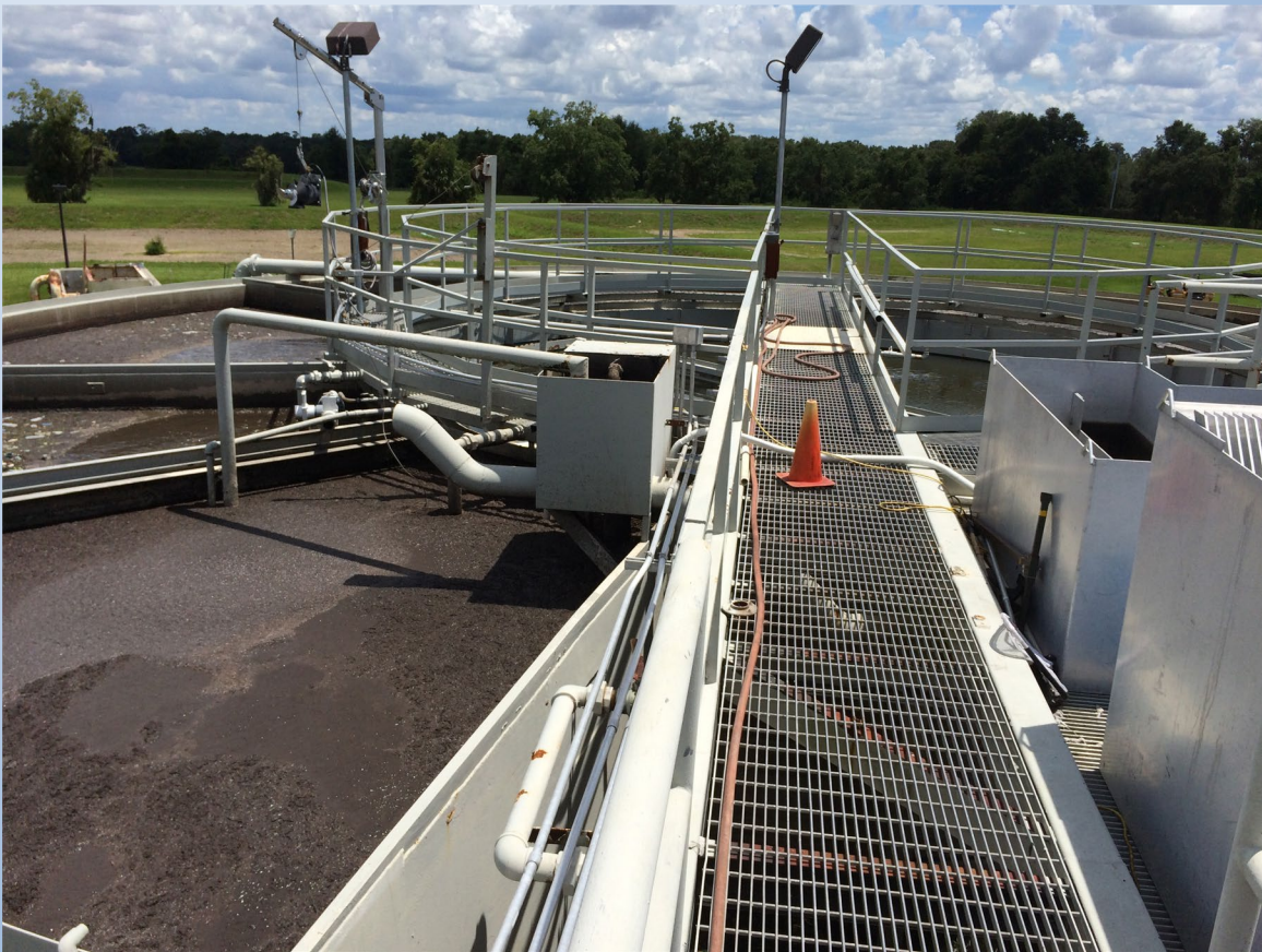
The City of Hawthorne Wastewater Treatment Facility
