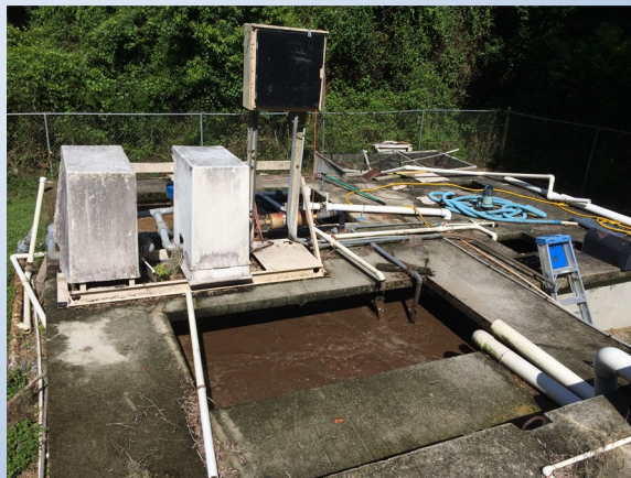
The Archer Homes WWTF
