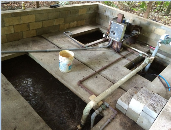
Camp McConnell/Cuscowilla aeration basin and clarifier
