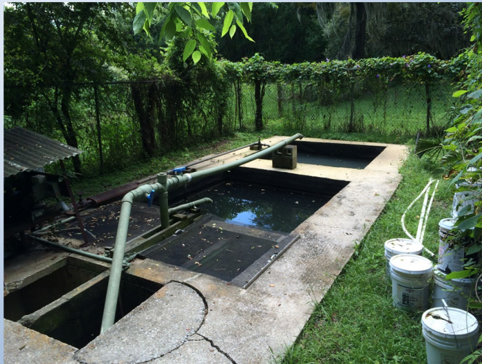
The Prairie View Apartments WWTF
