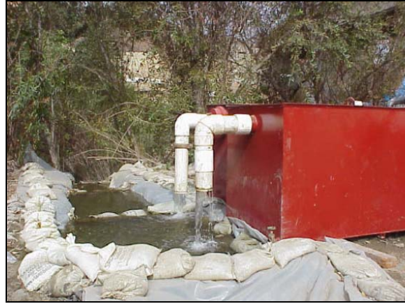
Dewatering Tank (Source: http://www.dot.ca.gov )
