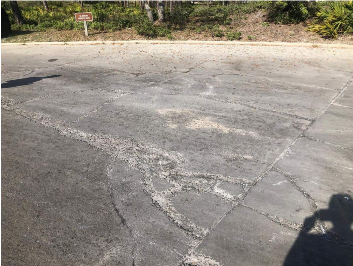
St. Andrews State Park P-8 - General Roadway Conditions
