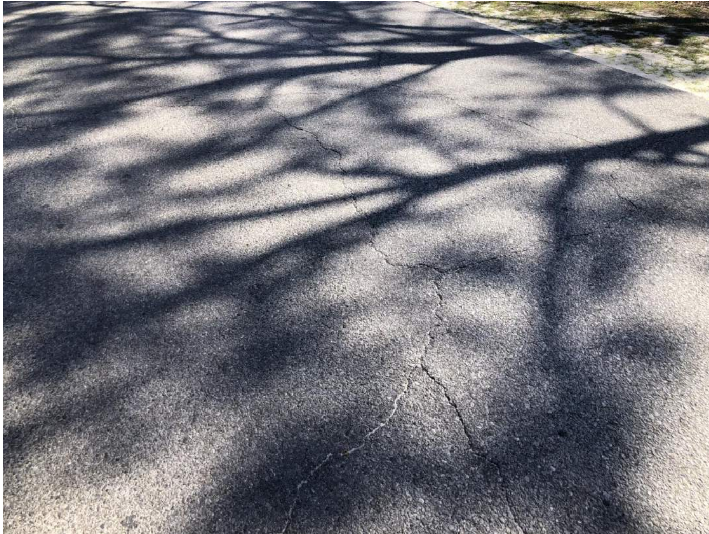
St. Andrews State Park P-7 - General Roadway Conditions
