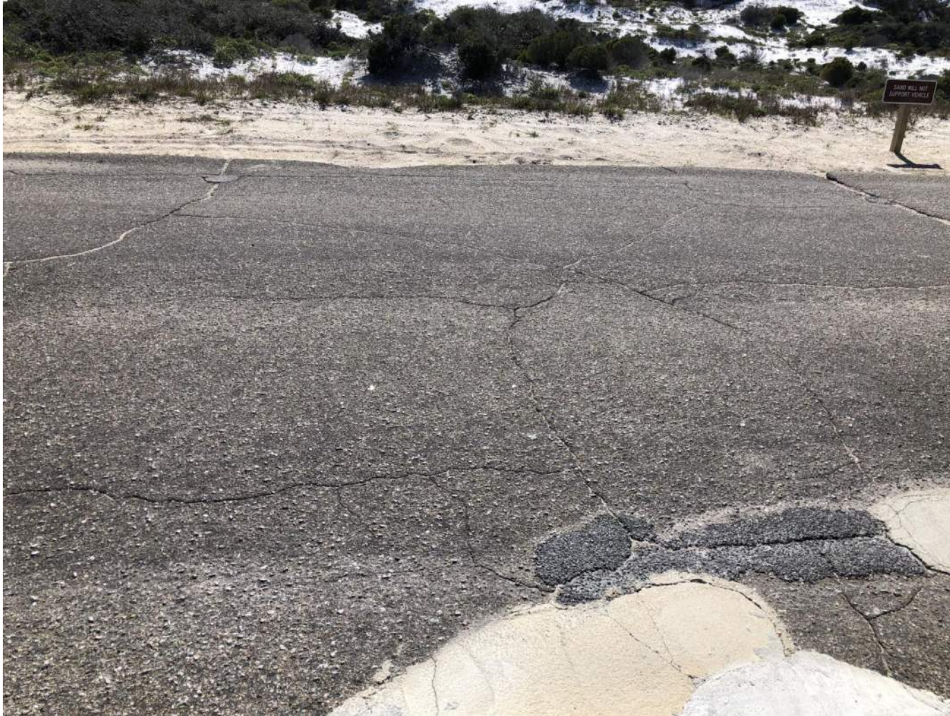
St. Andrews State Park P-2 - General Roadway Conditions
