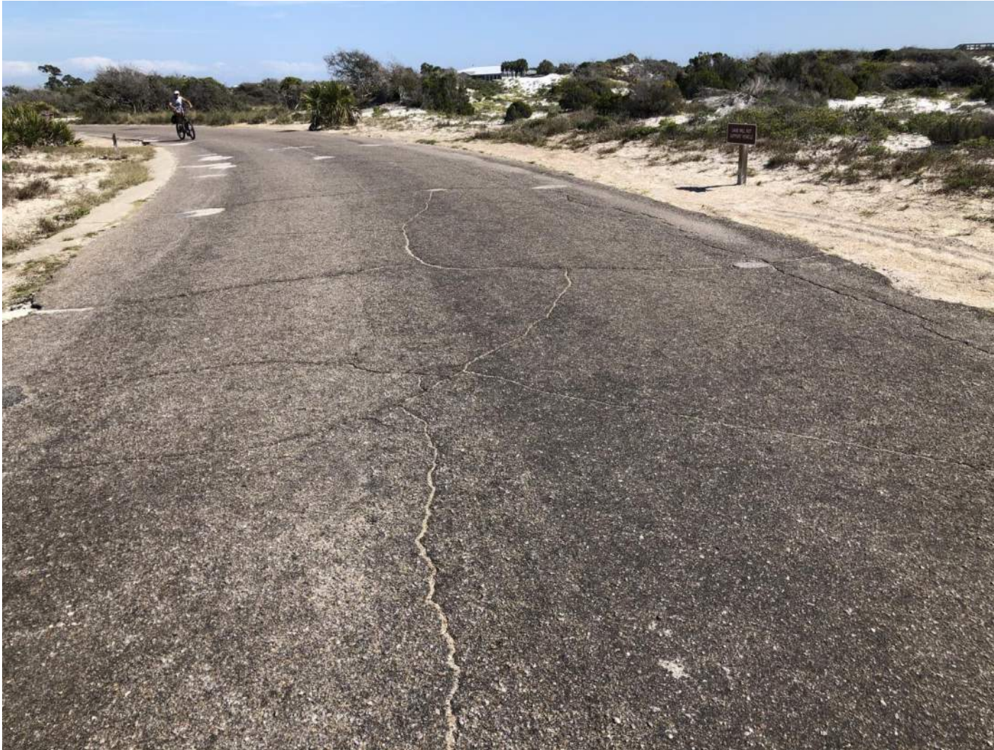
St. Andrews State Park P-4 - General Roadway Conditions
