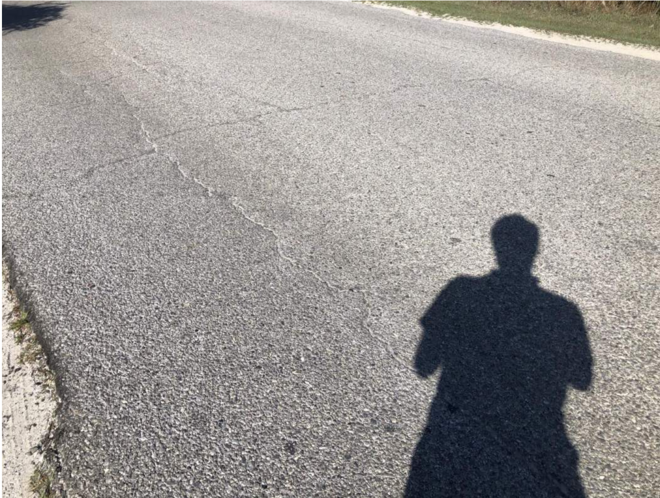
St. Andrews State Park P-1 - General Roadway Conditions
