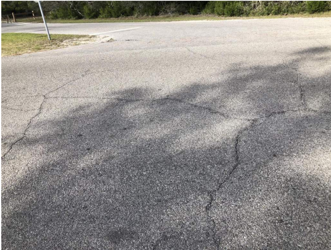
St. Andrews State Park P-6 - General Roadway Conditions
