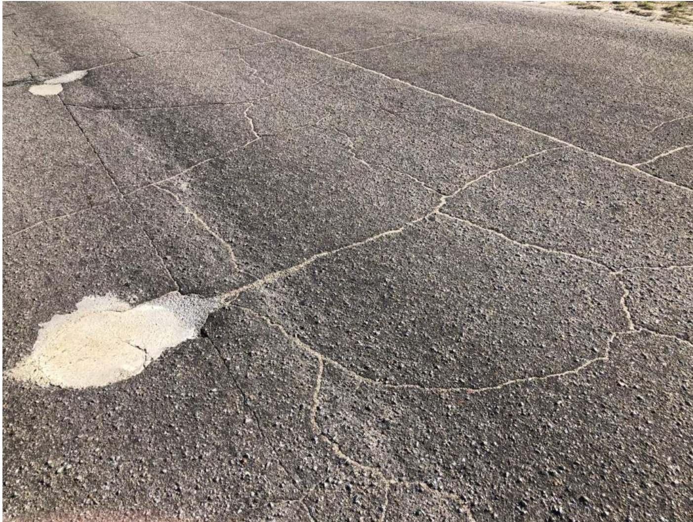
St. Andrews State Park P-3 - General Roadway Conditions
