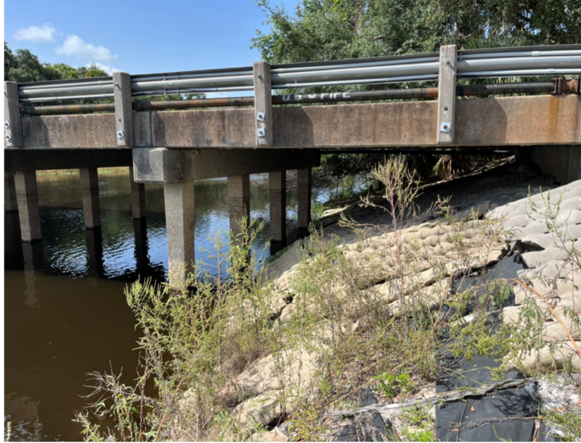
Figure 7 – Damaged Sand Cement riprap at West End Bent
