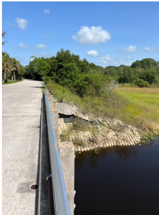
Figure 6 – Top of rail and bridge slab. Damaged Riprap at West End Bent
