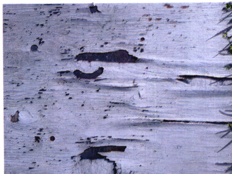
PHOTOGRAPH 6 Deterioration of wood sub floor
