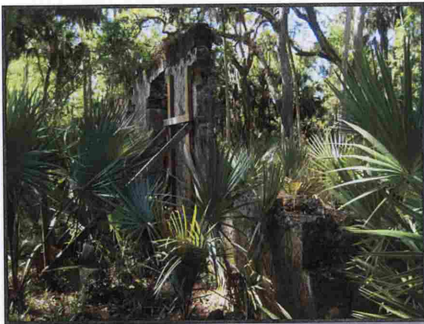
Figure 35. Structural bracing of extant wall elements at the Addison-MacRae Sugar mill feature (8VO7496) as noted during the GPS survey in April 2010
