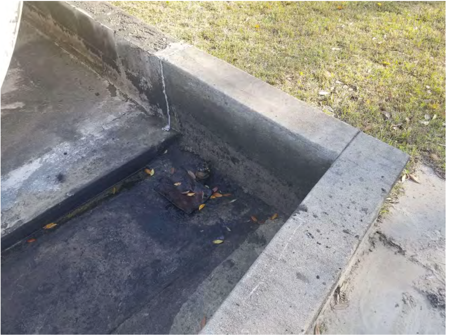
Figure 7: Rinse water drain area
