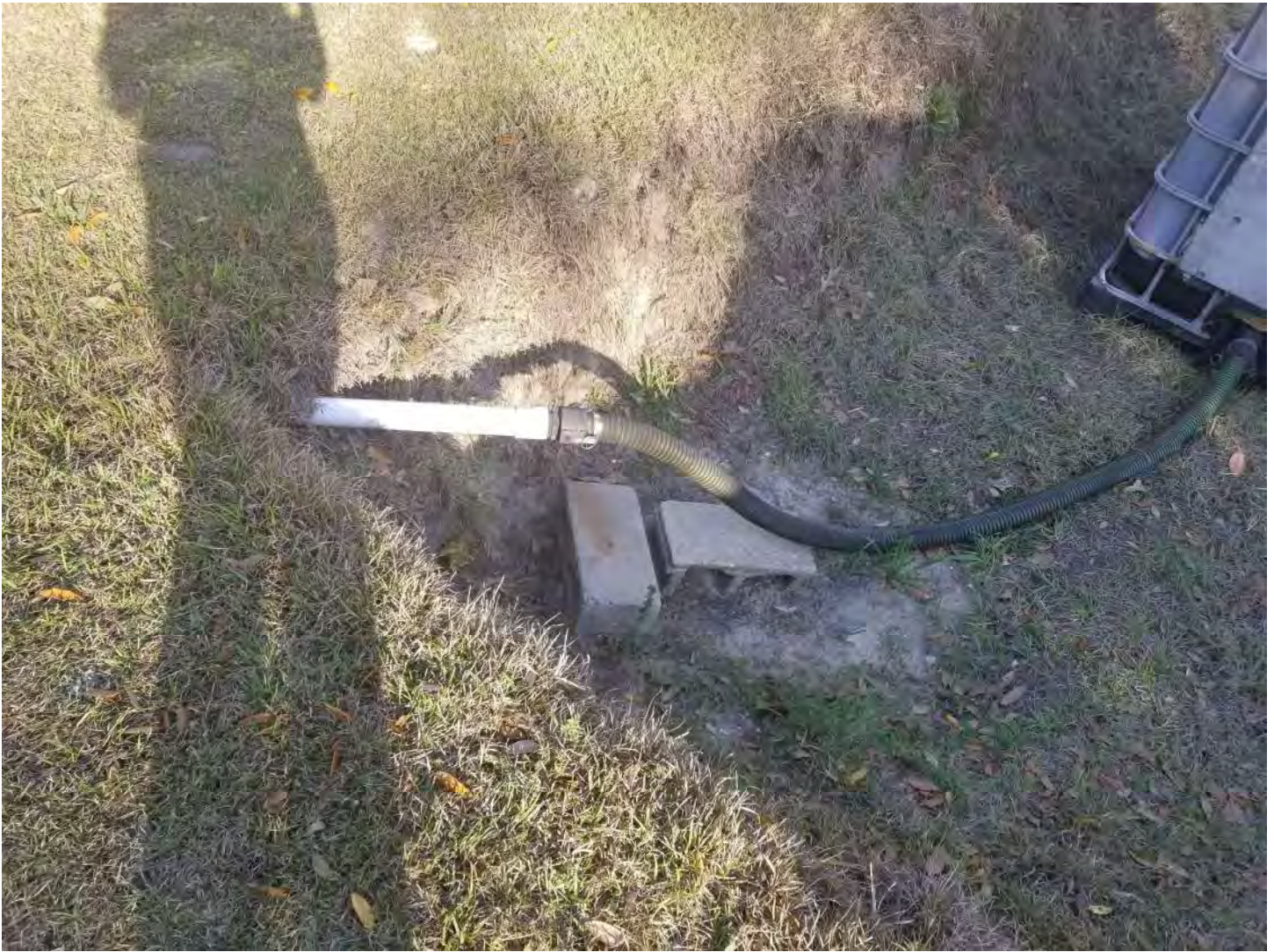
Figure 9: Rinse water drains to storm pond area where it is pumped to tanker truck
