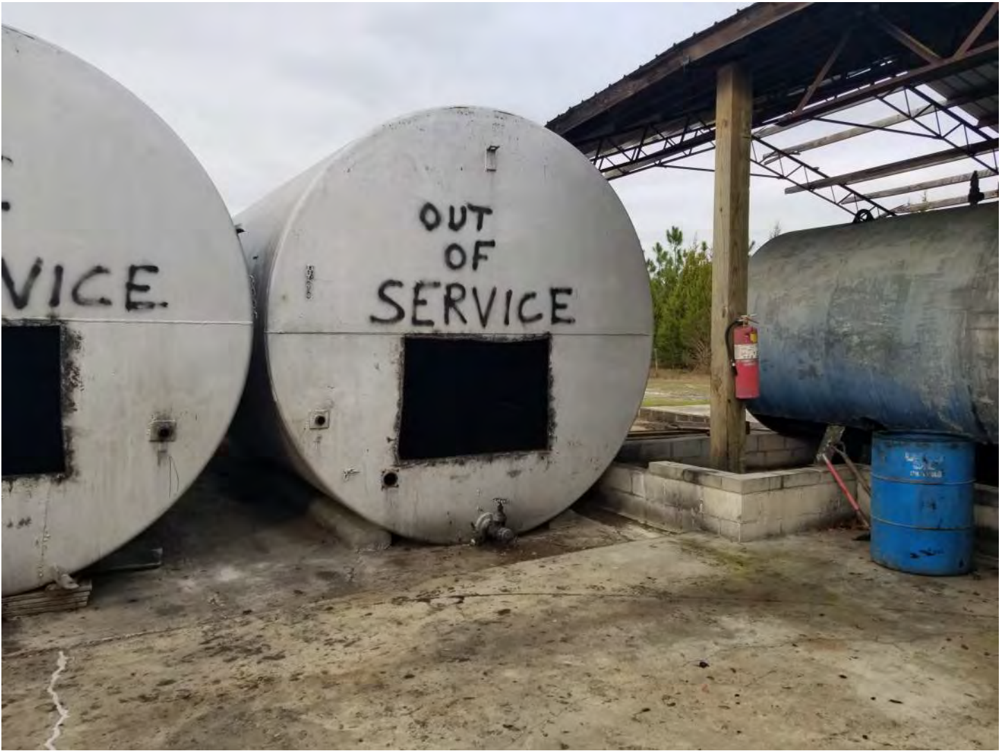
Figure 2: Tanks 2, 3, and side of boiler
