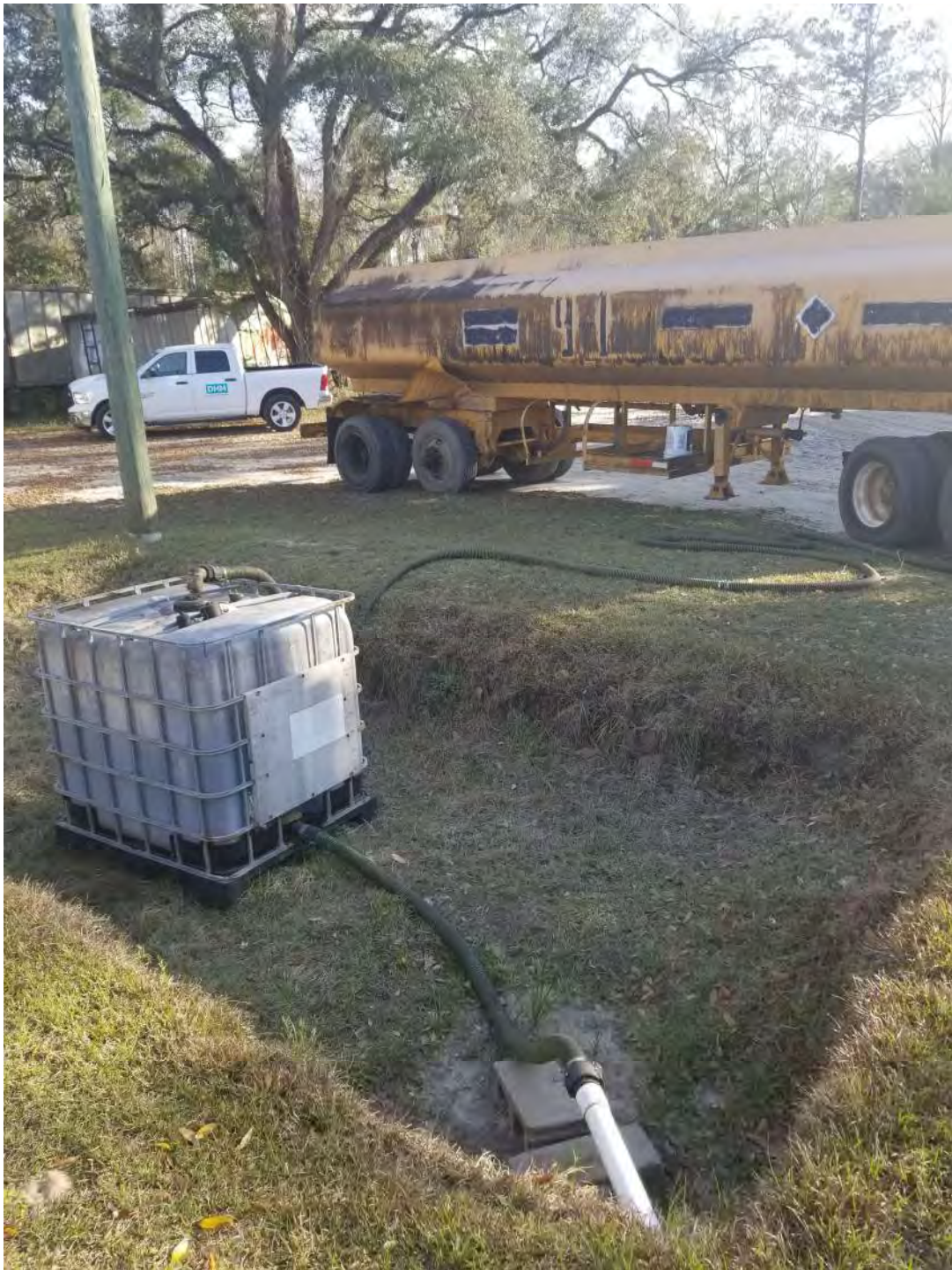
Figure 12: Rinse water drains to here where it is pumped to tanker
