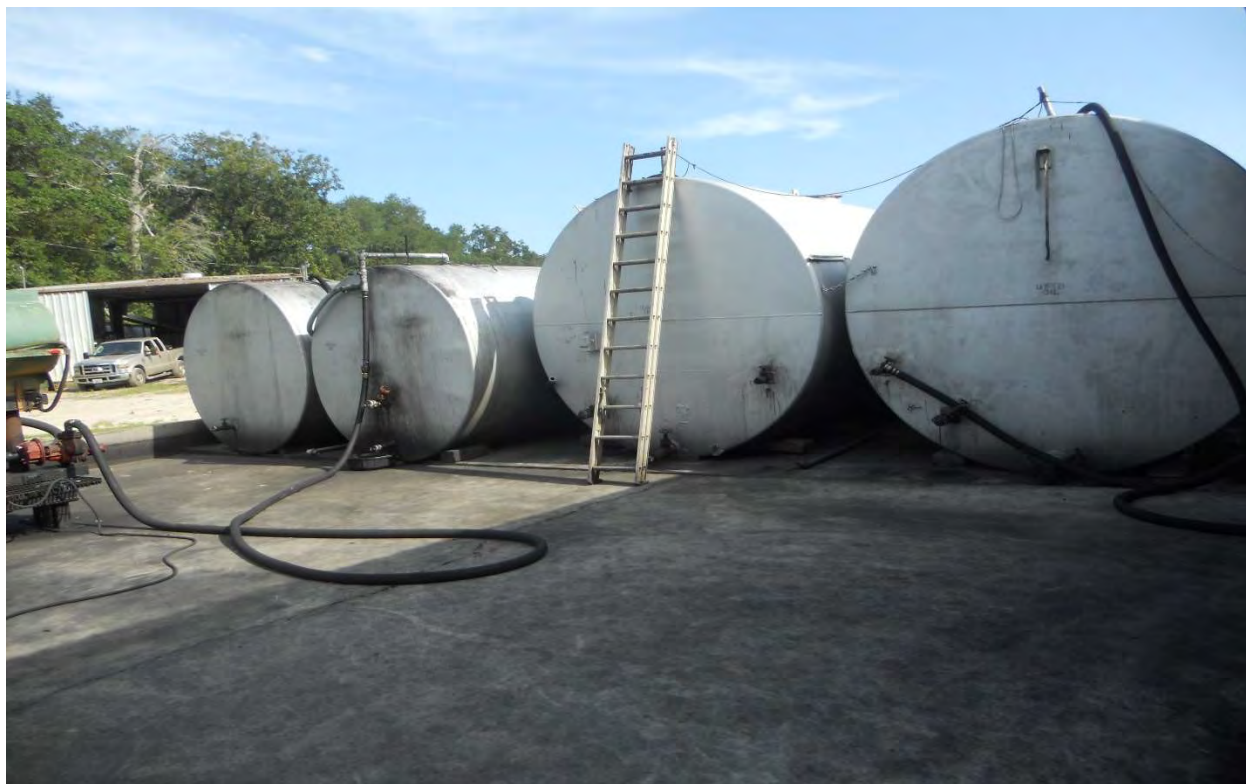
Storage Tanks within Containment Area
