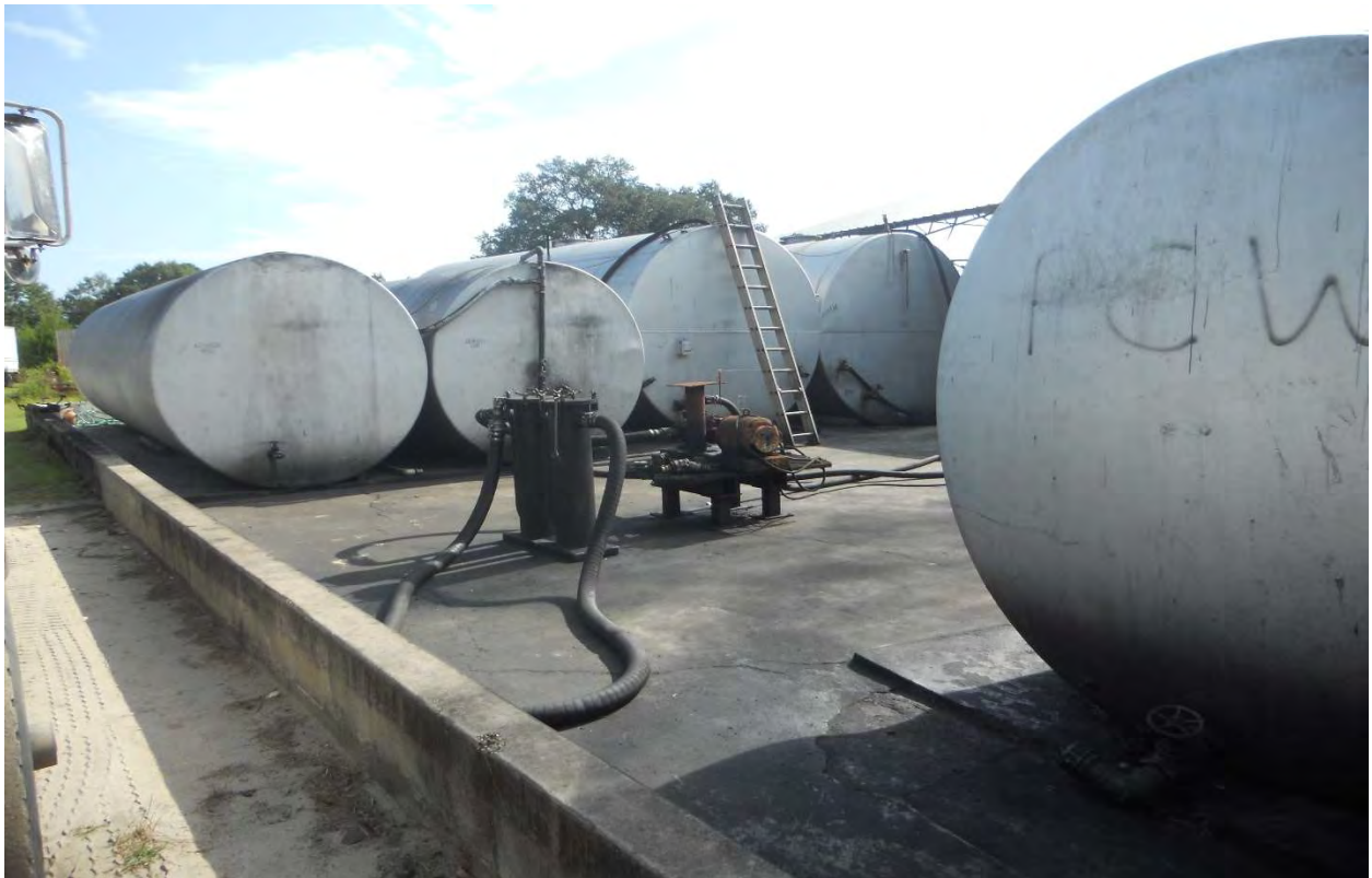
Storage Tanks within Containment Area
