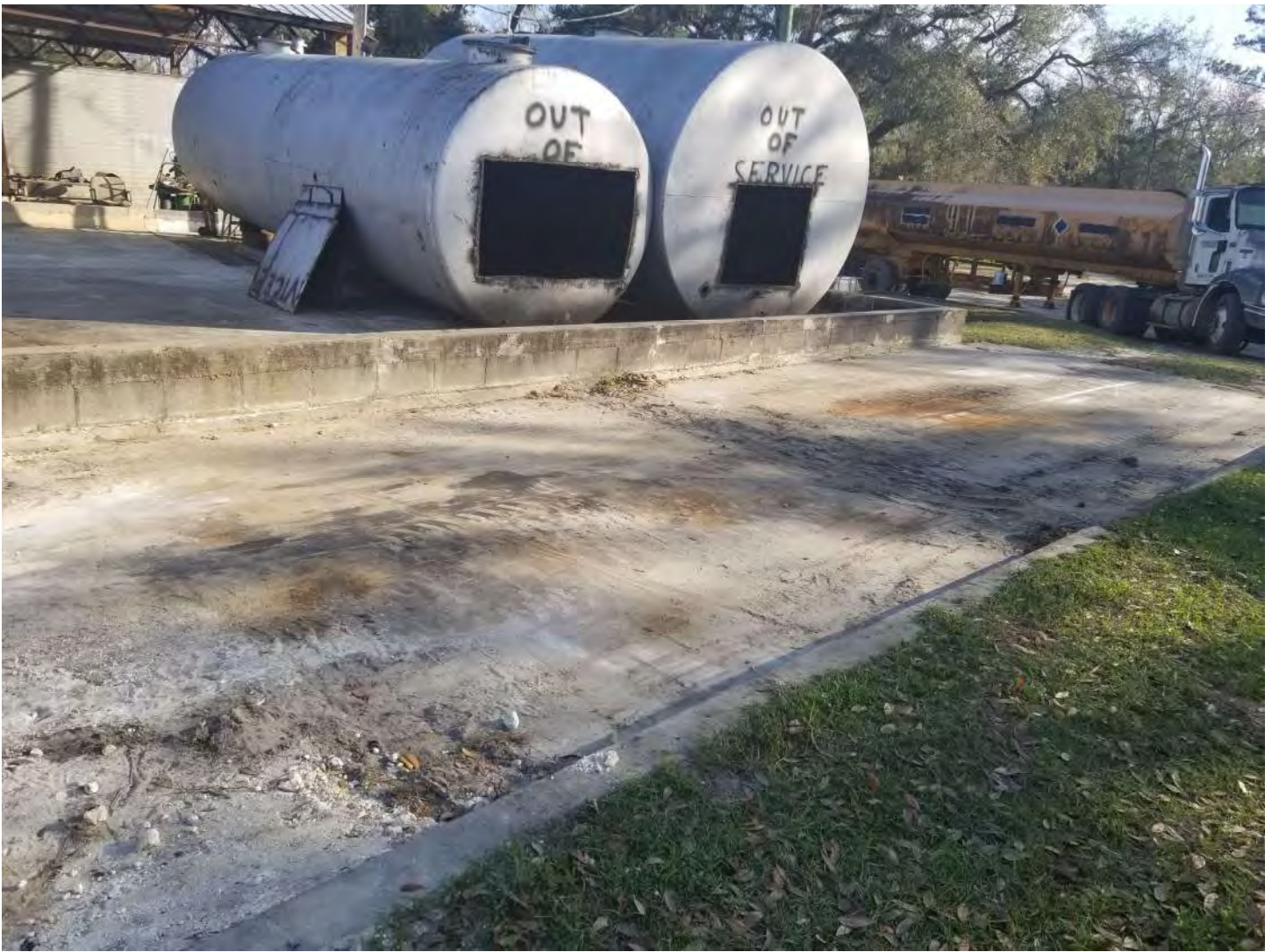
Figure 3: Tanks 3, 4, and tanker truck
