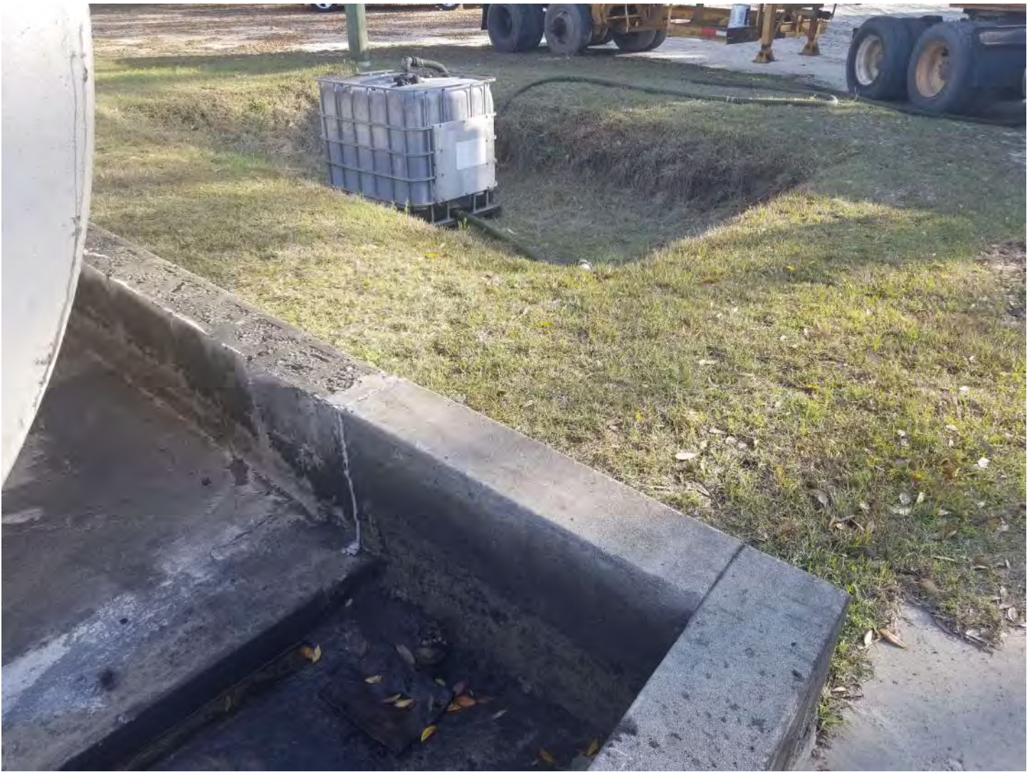
Figure 8: Rinse water drains from concrete storage area to the pump located in stormwater area
