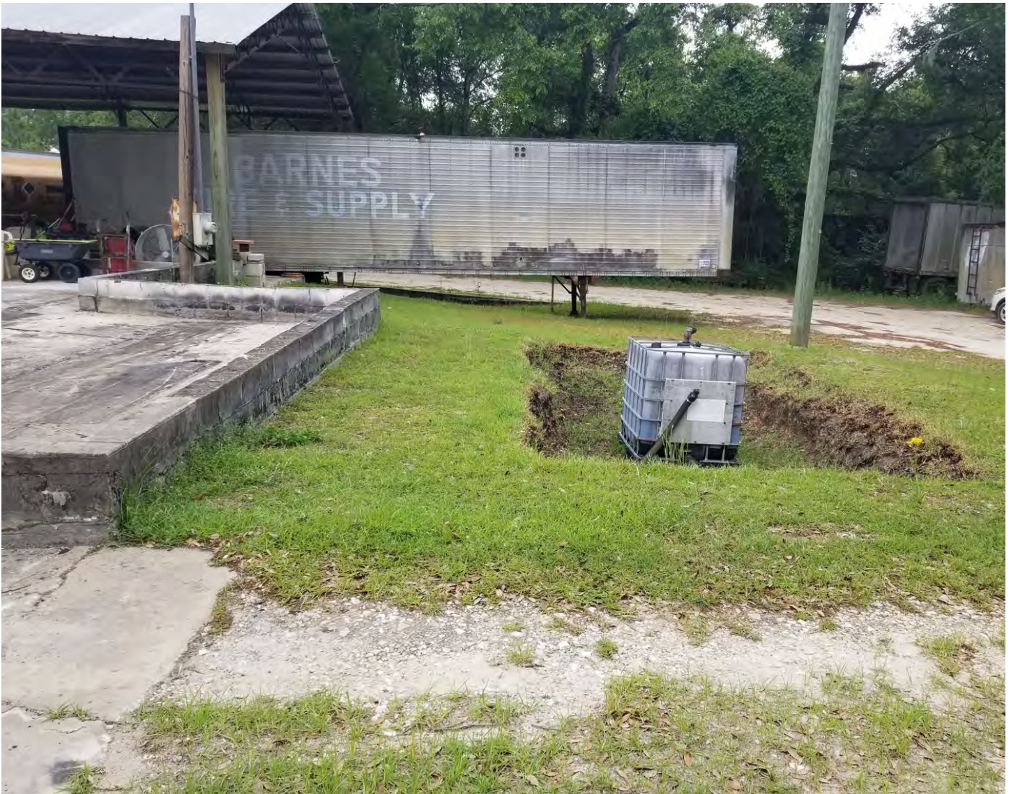
Figure 4: Stormwater Pond and pump
