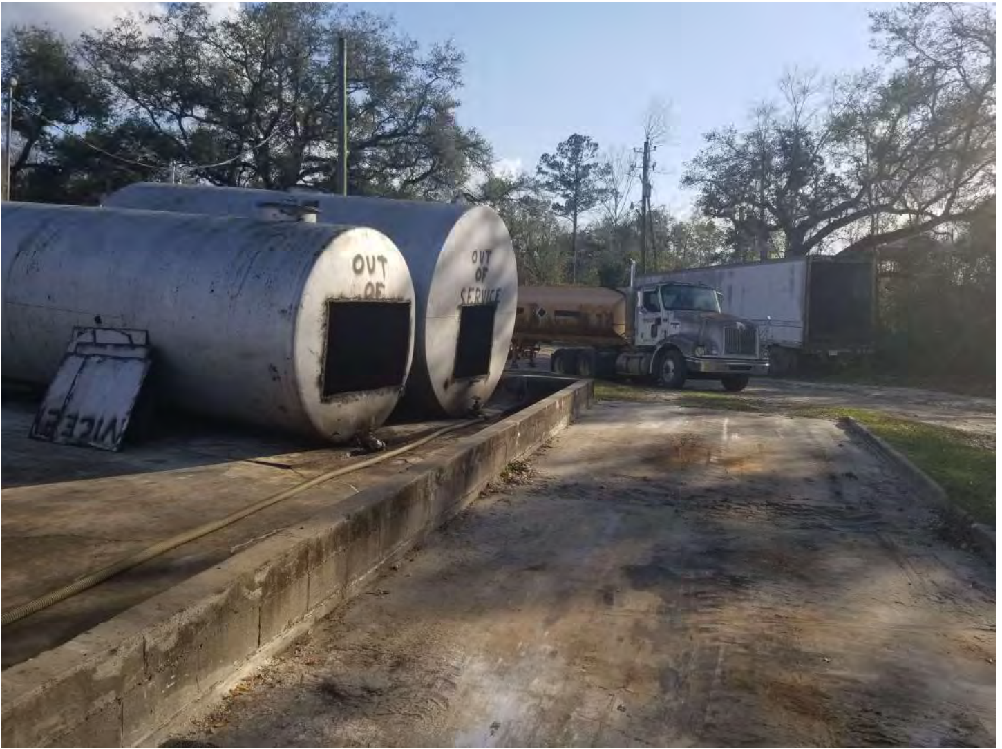
Figure 6: Rinse water drains through pipe to concrete storage area, then to pump located in storm drain area, and finally to tanker truck
