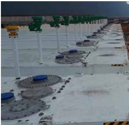
SOCOTTRA 1,320,860 USG fuel storage
