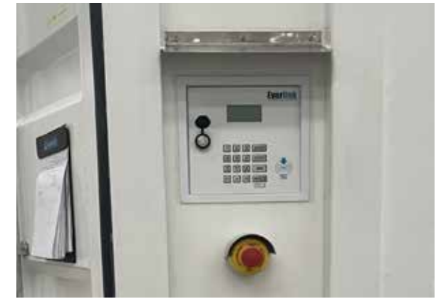
ADDITION OF FUEL MANAGEMENT SYSTEMS
