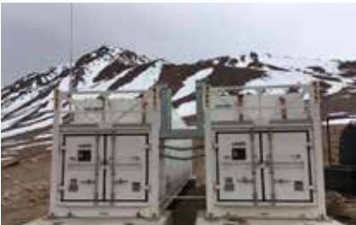
Remote Fuel Storage for Mine, Chile
