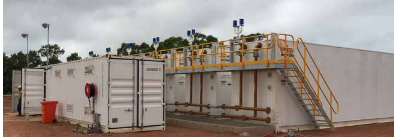
METRO MINING - 158,503 USG diesel fuel farm. 1x Adblue tank at remote site mine in North Queensland
