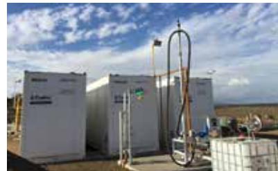
Mine Site Refuelling Facility Australia
