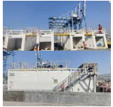
Fuel Depot for a Port in UAE 4xLTkB 47 – 2 hours Fire rated tank. Capacity – 12,416 USG GFL per tank
