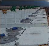
SOCOTTRA 1,320,860 USG fuel storage
