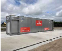
MODULAR FUEL STATION, UK
