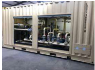
AVIATION MODULAR PUMP HOUSE
