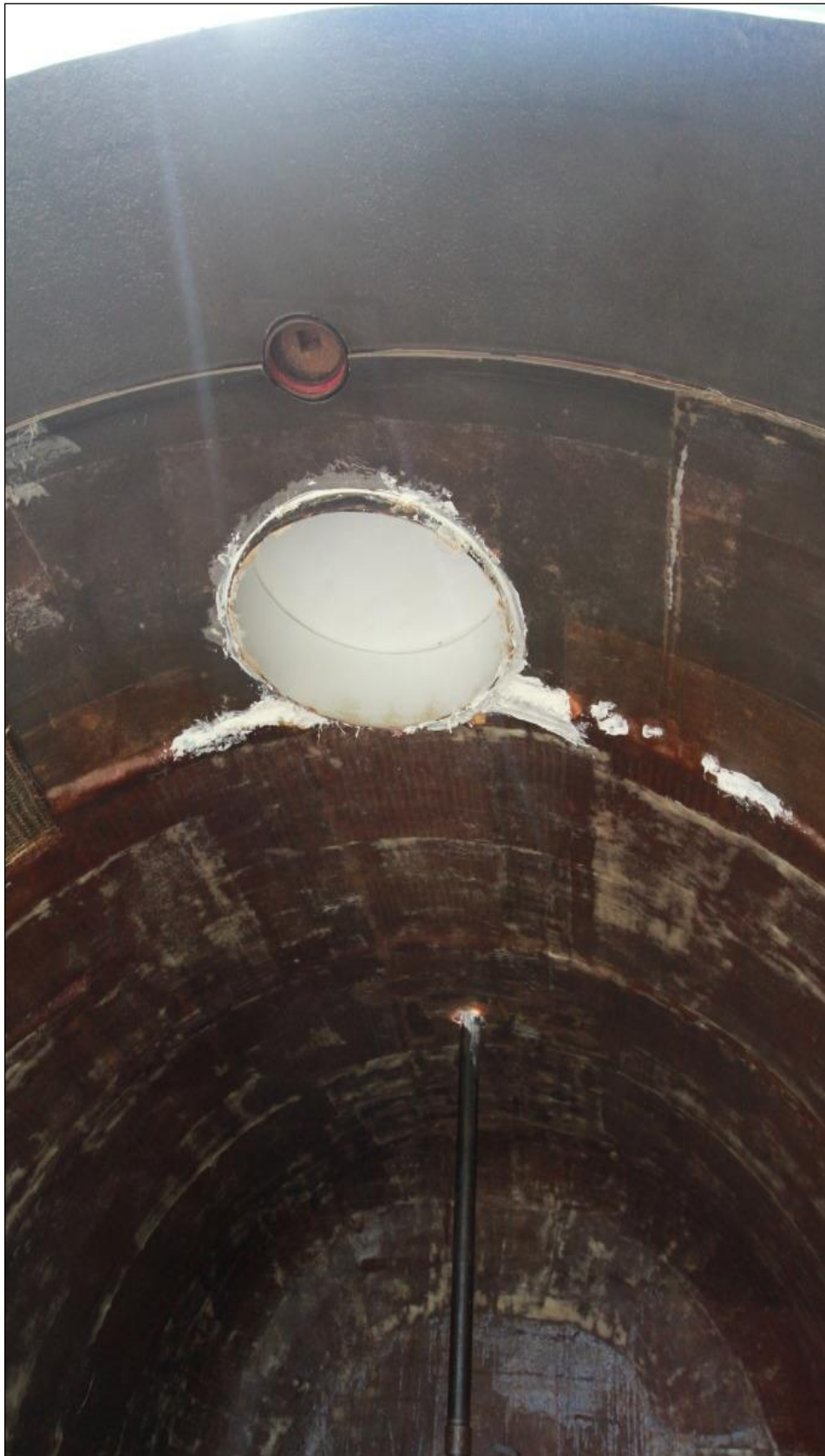
Figure 4. Interior of Tank Showing Manway and monitoring tube.
