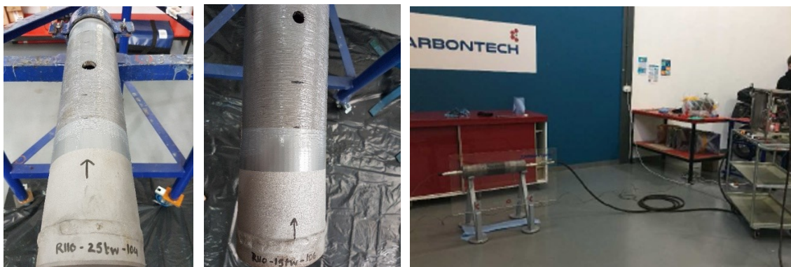
Figures 9,10 and 11: 25mm and 15mm defects before repair, testing of repaired spool
