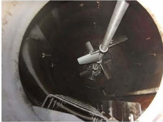
Figure 4. The Internal of the Tested Vessel
