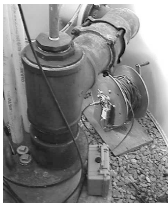
FIGURE 6. Fountain Hill's ASR well. View of well from inside the vault. (Photo courtesy of HydroSystems, Inc.)
