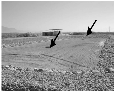
FIGURE 4. Basin 2 at The Superstition Mountain Community Facility District #1 Recharge Facility. Vadose zone wells 3 and 4 are located within the basin in the foreground and background respectively. (Photo by ADWR, 2005)
