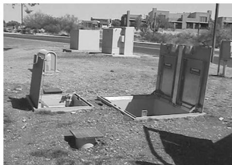
FIGURE 7. Fountain Hill's ASR completed vault to well which is located underground. (Photo courtesy of HydroSystems, Inc.)
