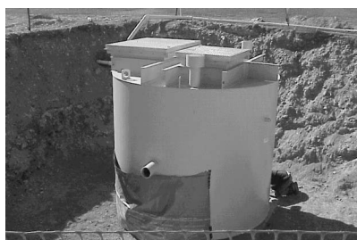
Photo 2. Well and concrete pad housed inside vault.
